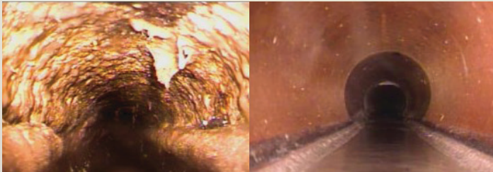
A grease clogged sewer pipe: Before & After
