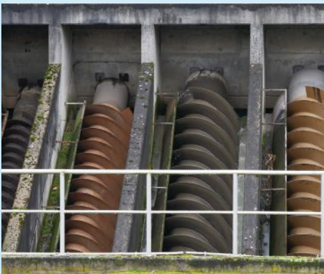
The water station's maintenance team applied Chockfast to support the mounting bars, and all repaired and new gearboxes.
