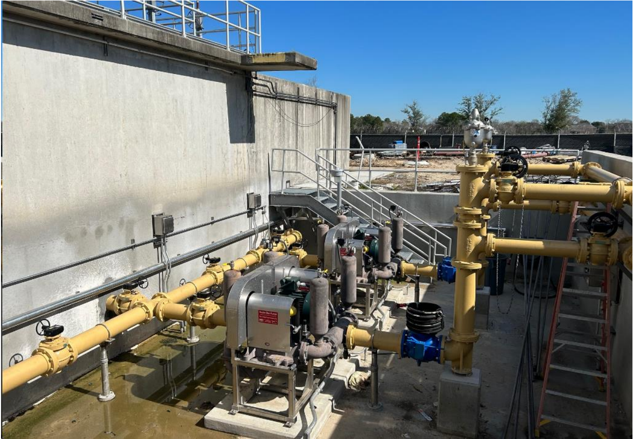
Aerated Holding Tanks
