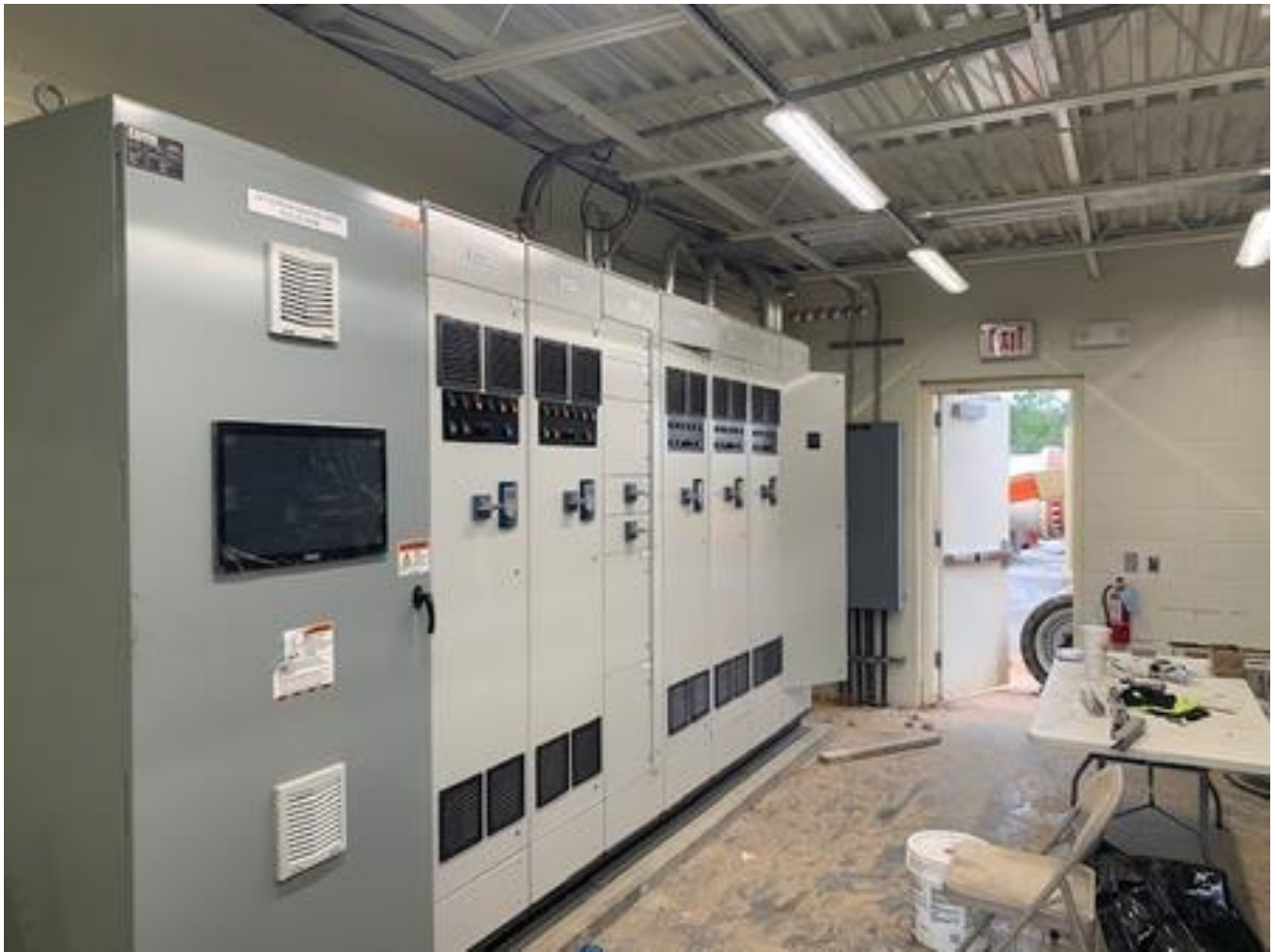
Motor Control Center (MCC) 2
