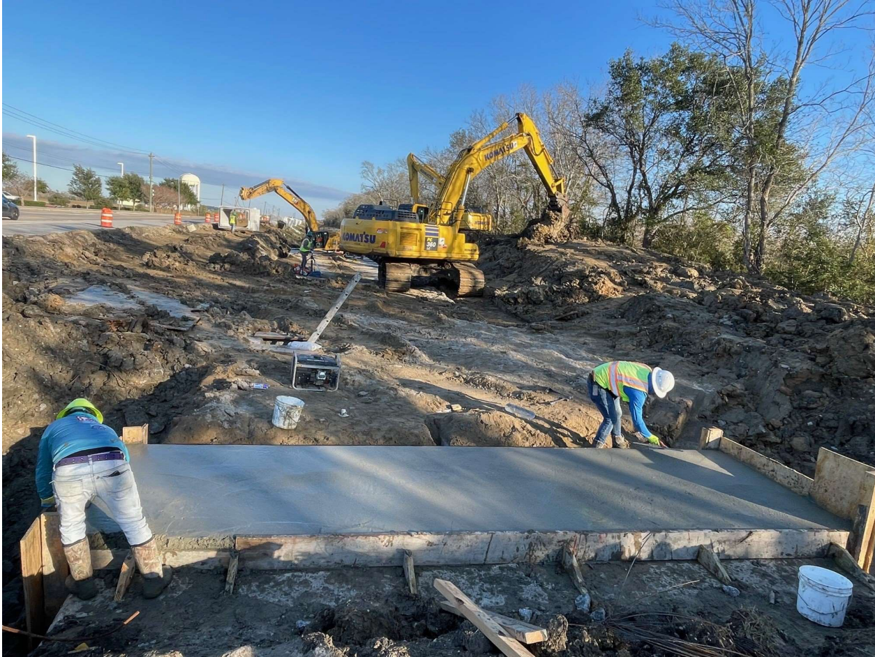
Connecting existing storm pipes to new 8'x5' Reinforced Concrete Boxes near Bailey Road/Veterans Drive intersection
