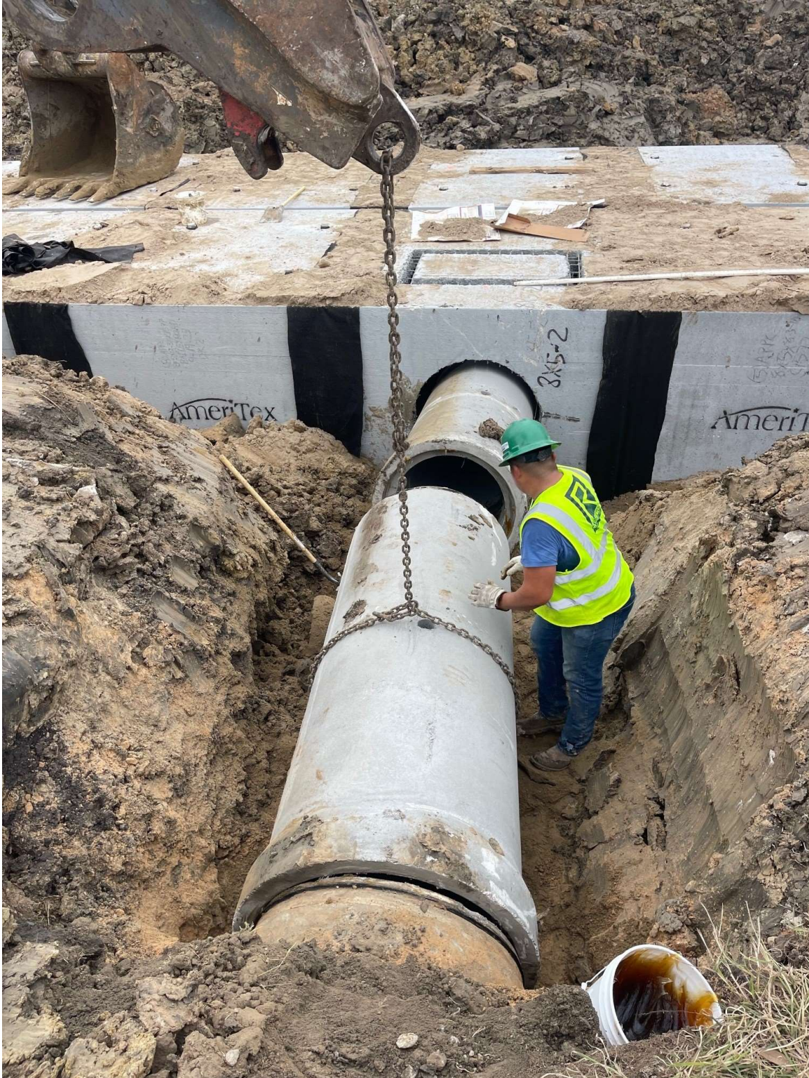
Installing new storm lateral pipe to new 8'x5' Reinforced Concrete Boxes storm pipe
