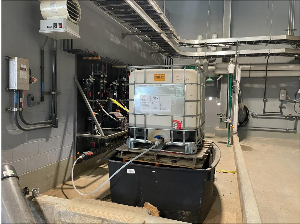
Temporary ACH tote chemical feed setup for making settled water
