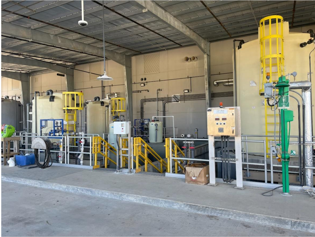
Chemical offloading area with eyewash and hose reels
