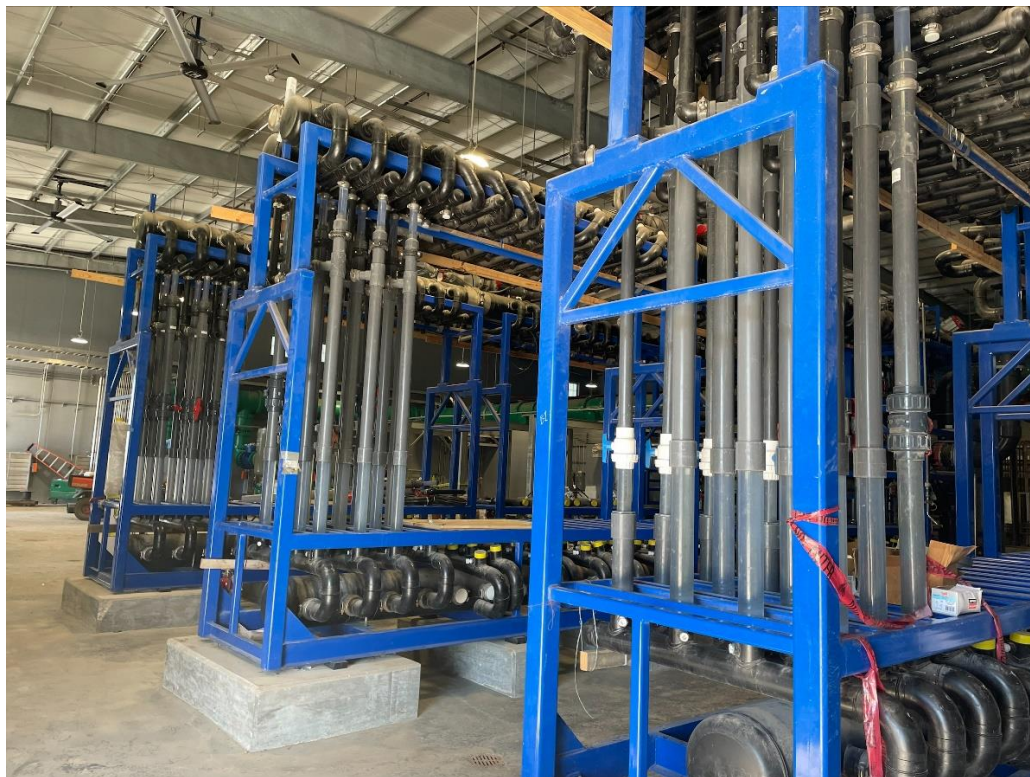
Dummy modules in membrane racks for system function testing
