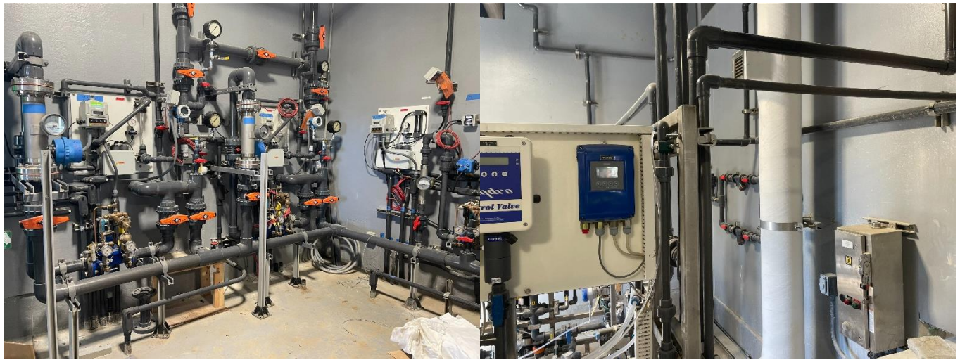
Chlorine Gas and Chlorine Dioxide Generator Piping
