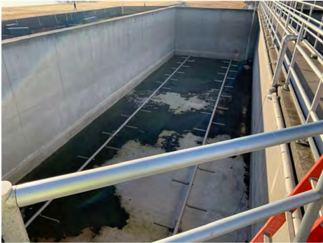
Aeriated Sludge Holding Tank (ASHT)
