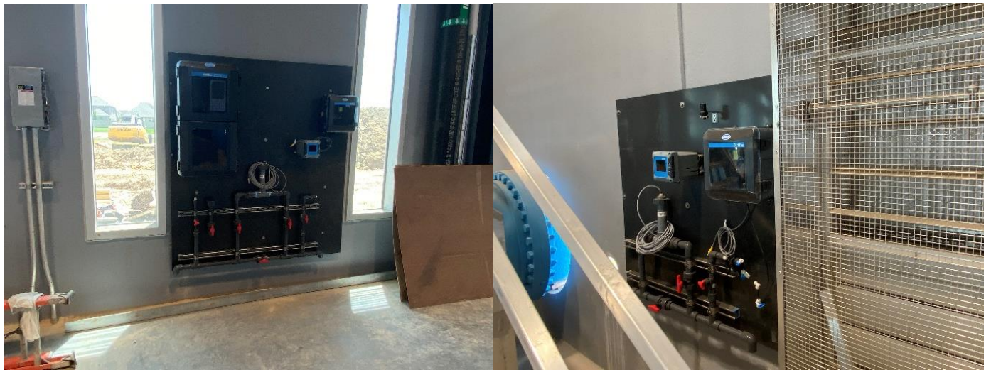
Analyzer installations in High Service Pumping Station
