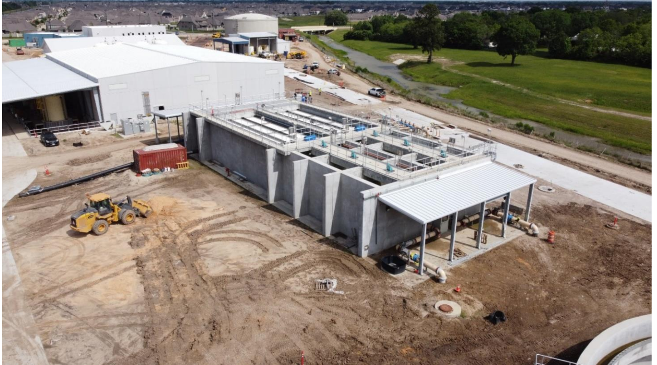
PreTreatment Unit with Flocculation Cells in foreground & Plate Settlers in background
