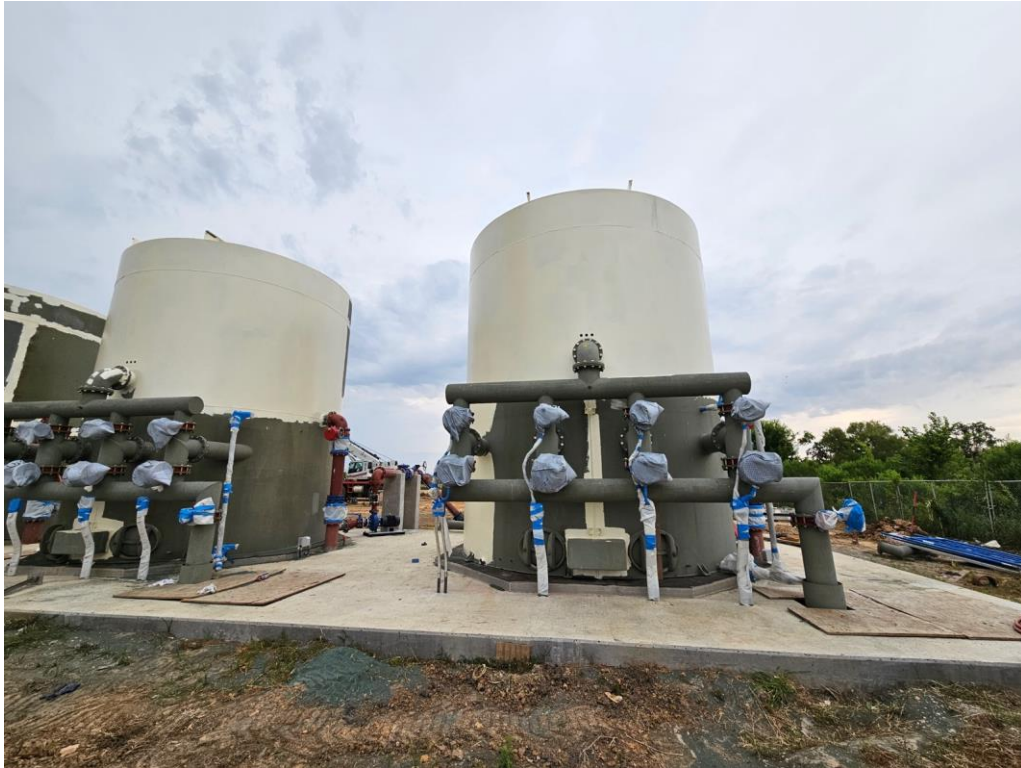
Pumps and piping for the aerators that treat the water from Magnolia Well
