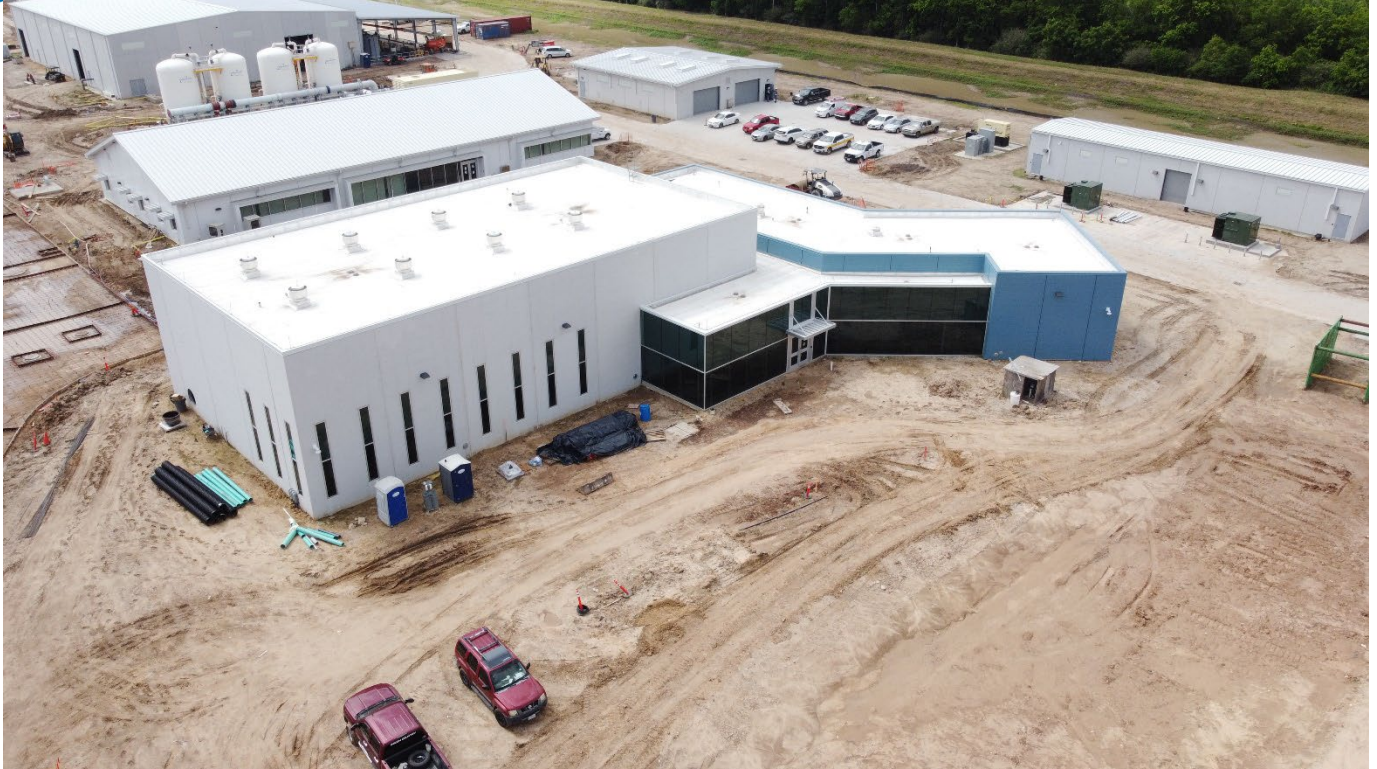
Public facing view of the plant, Administration and High Service Pump Building
