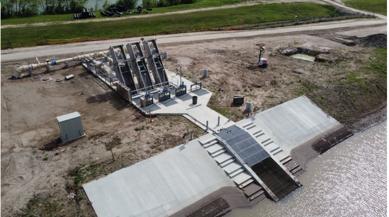
Raw Water Lift Station with Vertical Screens and Main Influent line in background
