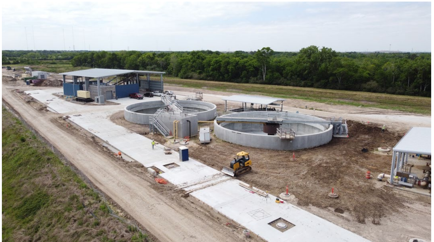
WashWater Recovery & Gravity Thickener
