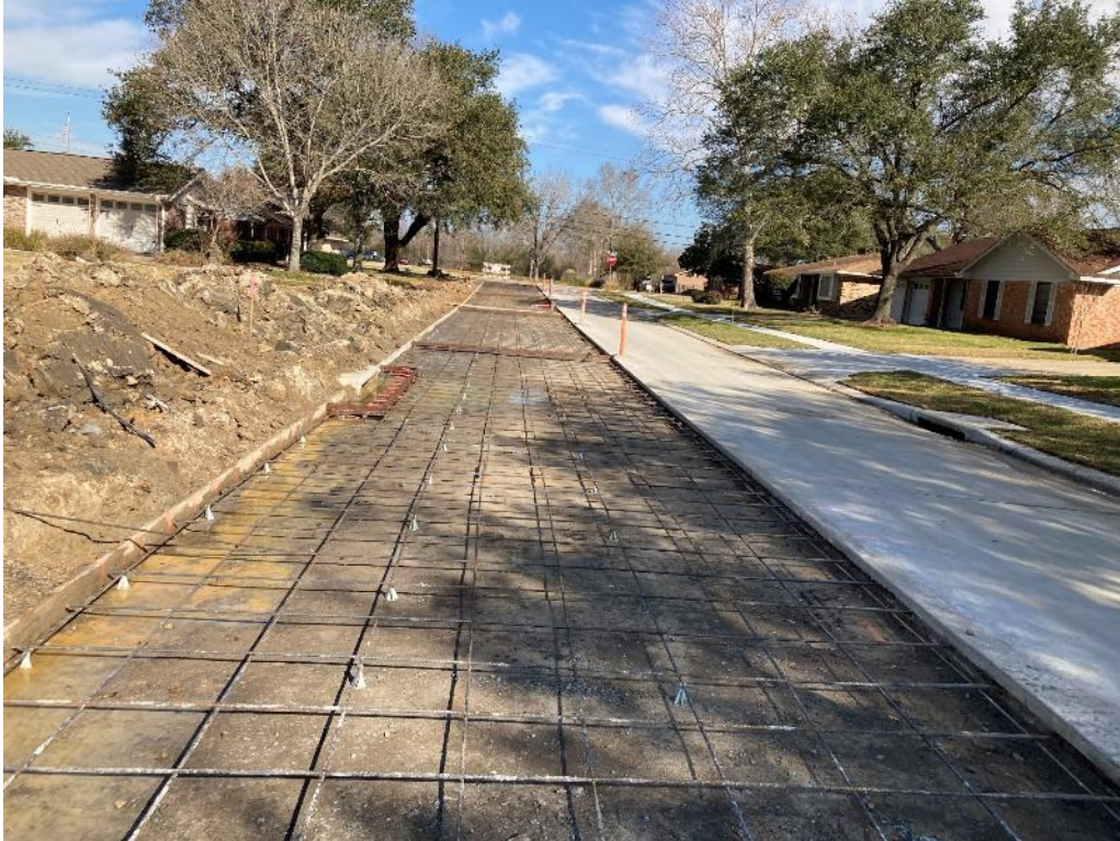
Forms and Steel for Paving on the West Side of Willow Blvd
