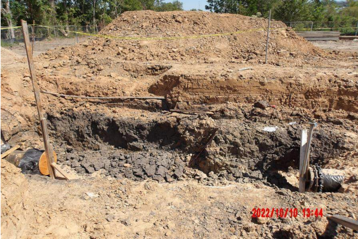
The End of the Magnolia Transmission Line and the Future Connection at Bailey WTP
