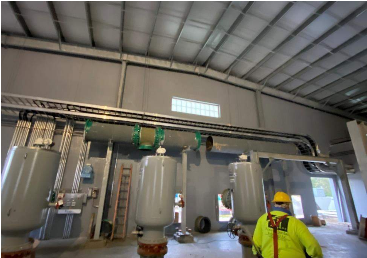
Pre-Membrane Strainers installed inside Membrane Bldg.
