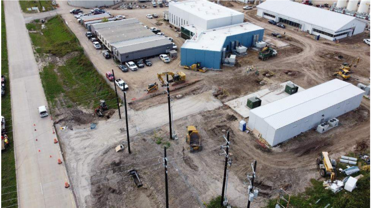
Initial subgrade preparation at Plant Entrance in preparation for beginning Plant Roadway Paving
