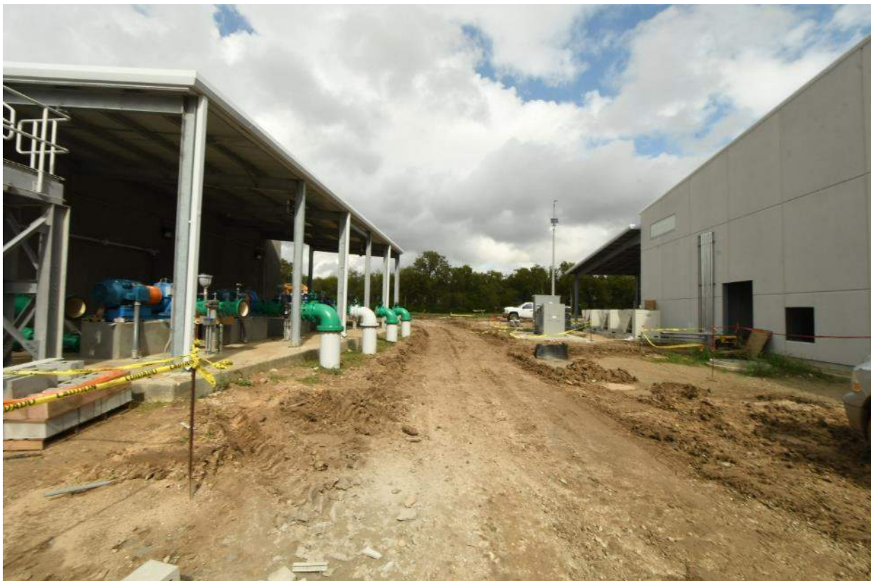
Feed Piping Settled Water from Pre-Treatment to Membrane Bldg.
