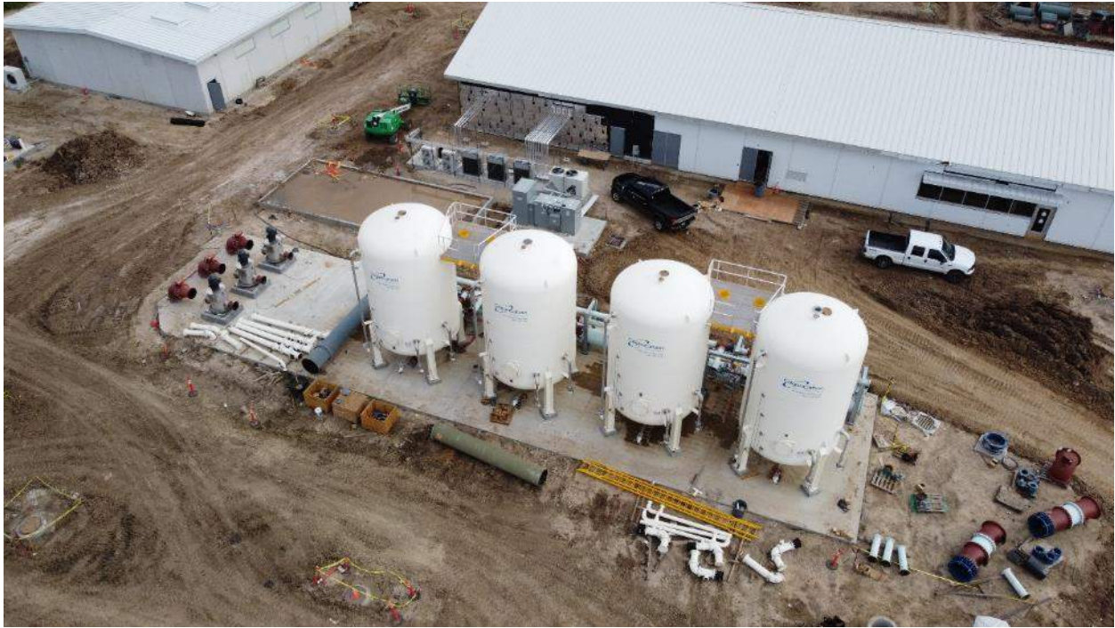
GAC Reactors and Piping
