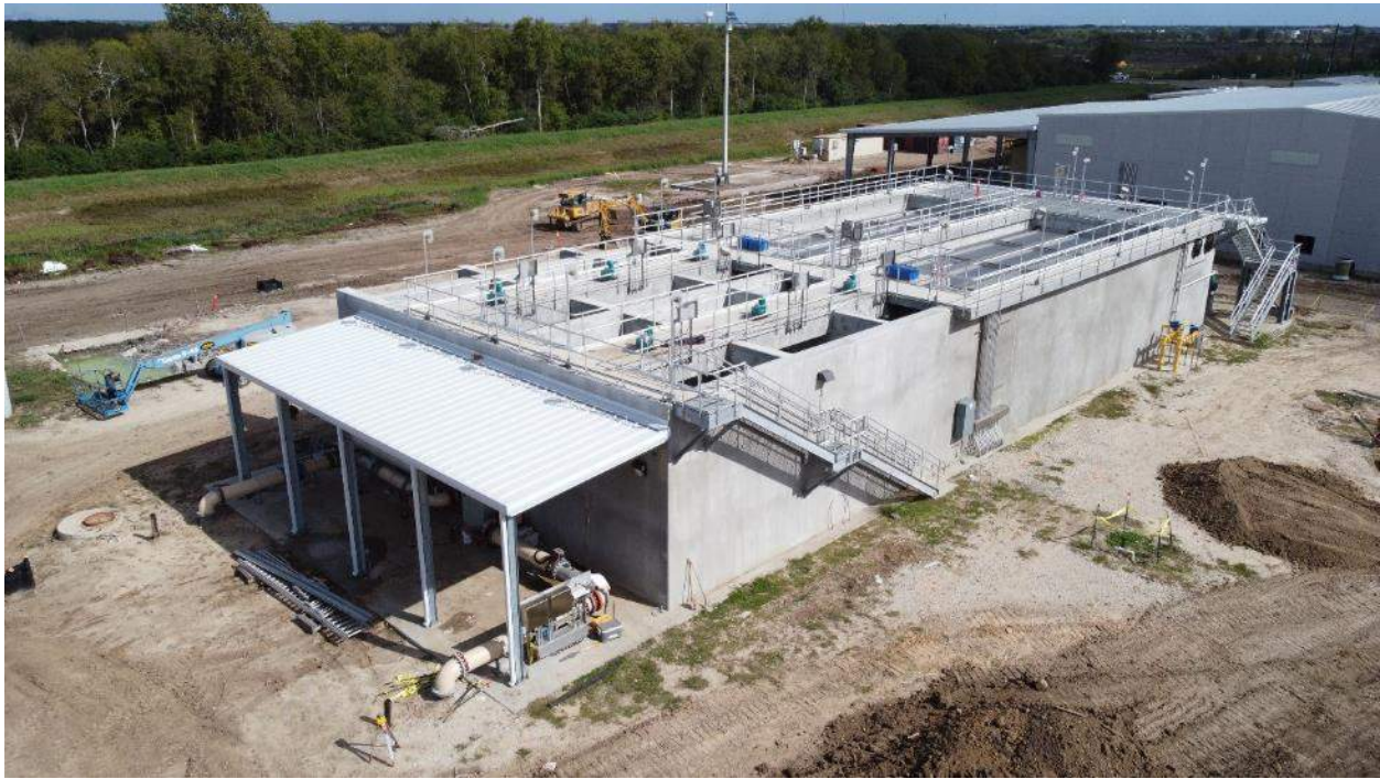
Raw Water end of Pre-Treatment showing supply piping for two settling trains
