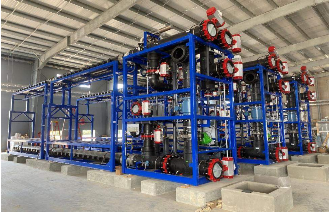
Membrane Racks awaiting the installation of Membrane Modules
