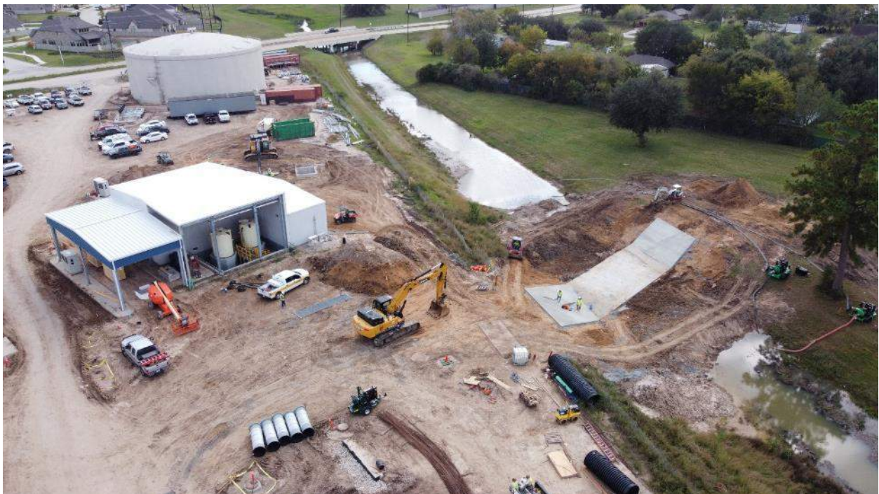
Chlorine Bldg with site drainage outfall in construction inside Mustang Bayou on right
