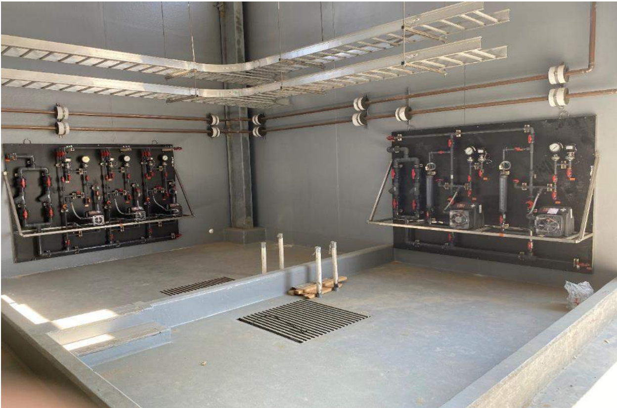
Chemical Feed Pumps for Membrane cleaning
