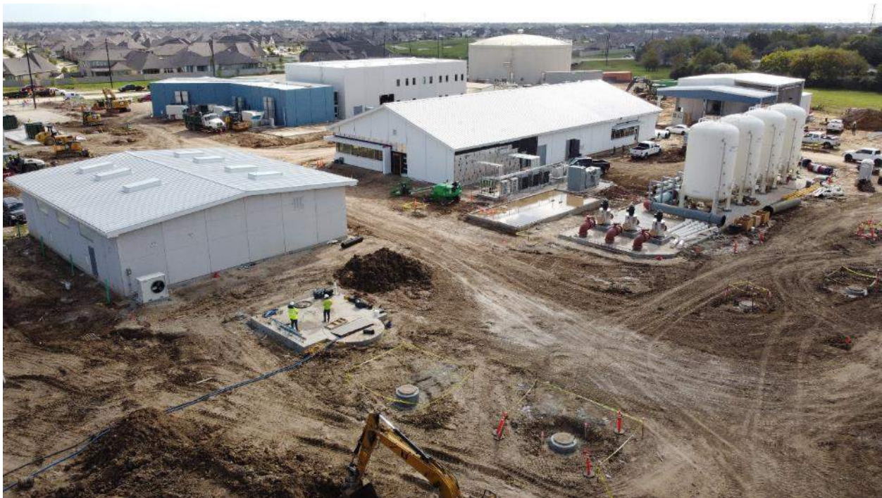
Site showing Sanitary Lift Station in foreground Maintenance Bldg. far left Operations and GAC far right and Admin/ High Service Pump Bldg. in background
