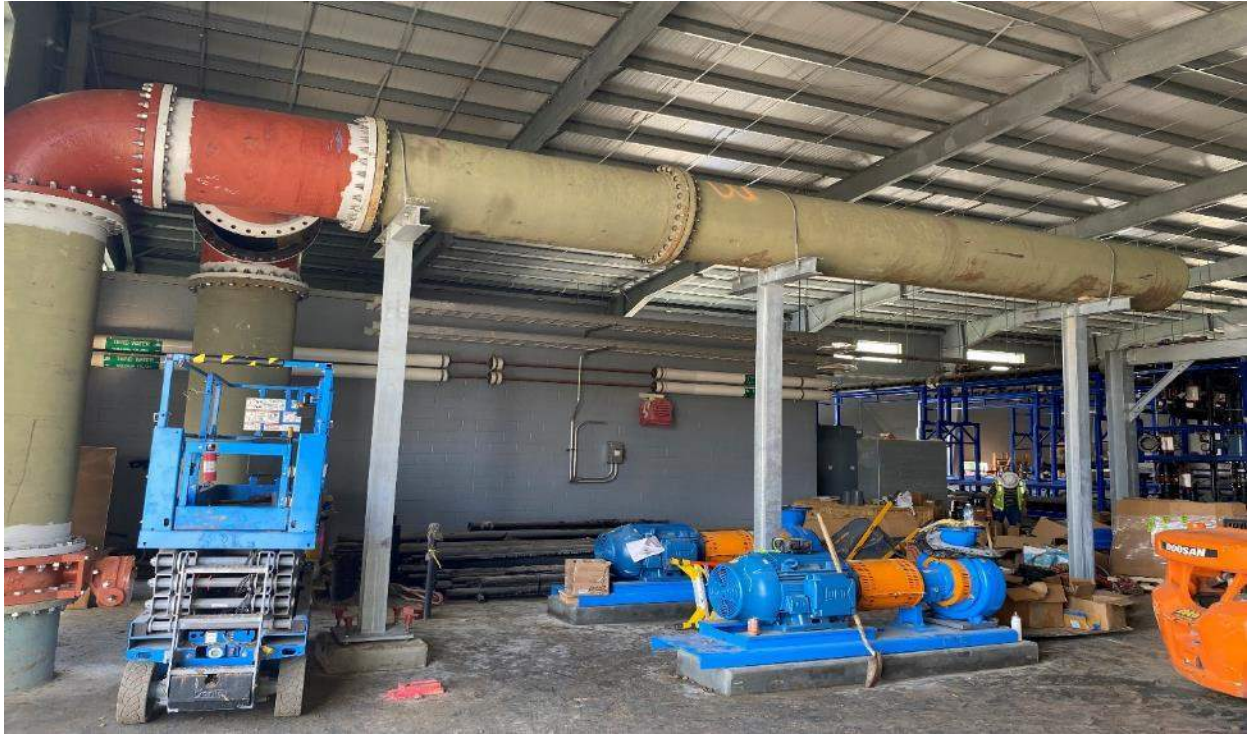
Water piping to/ from membrane racks
