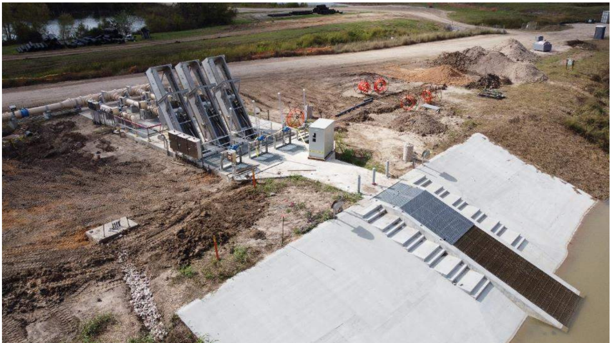
Raw Water Lift Station showing Intake Strainer and Vertical Screens
