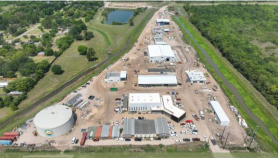
Surface Water Treatment Plant Operational in FY23 $175.5M - Construction in Process at 75%
