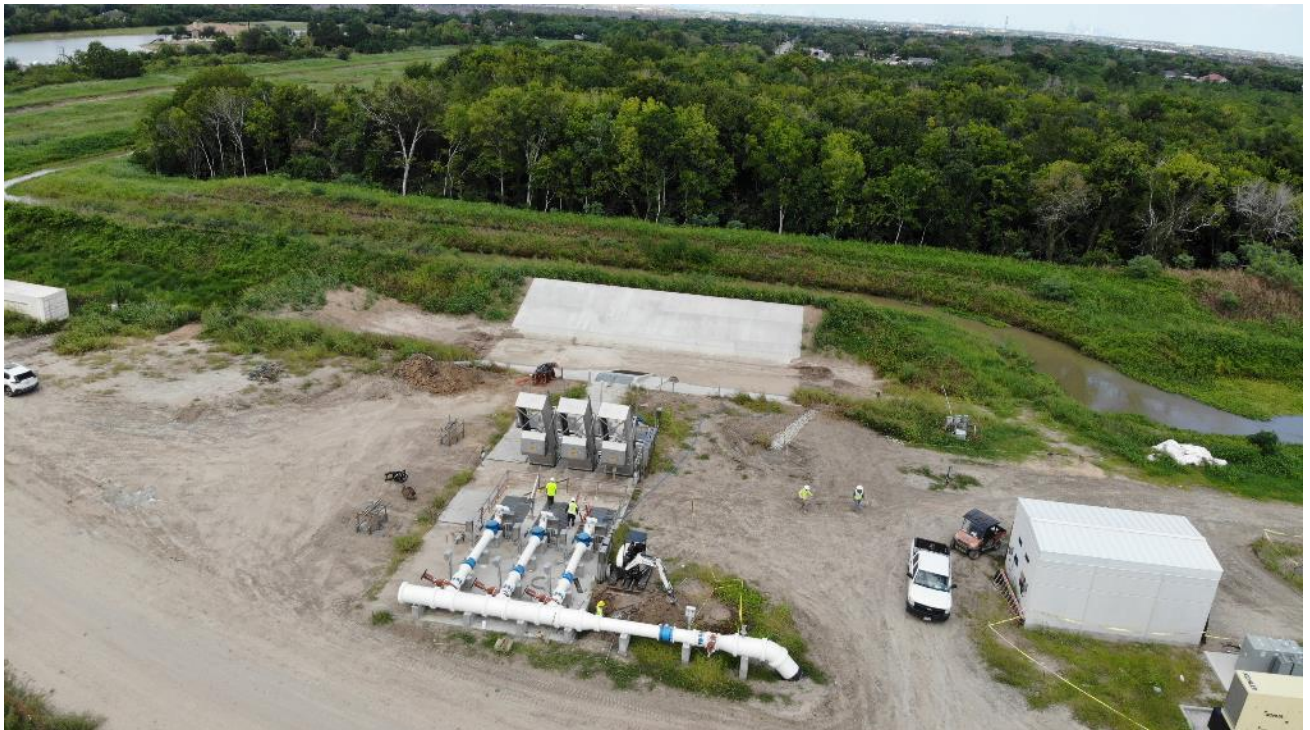
View looking North at the Raw Water Pump Station
