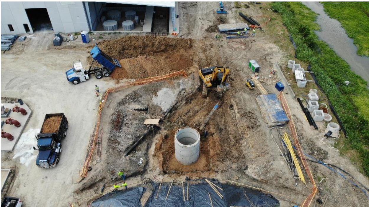
Sanitary Lift Station to service the Plant
