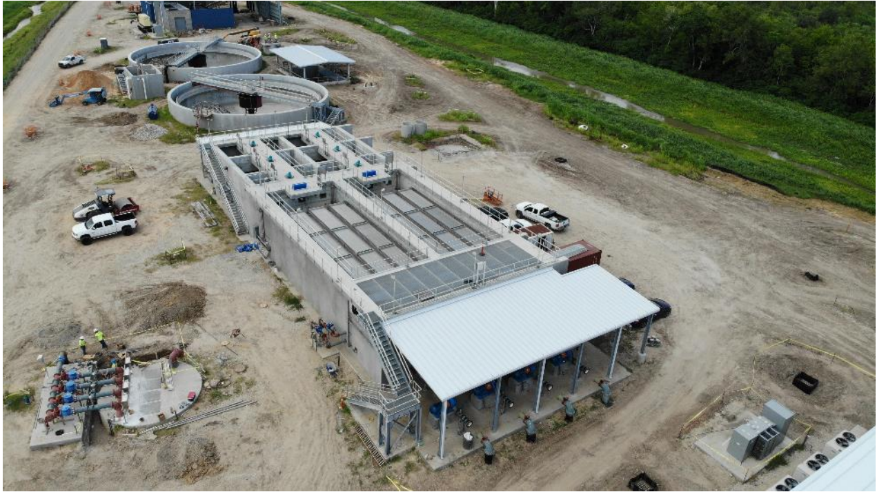
View of the Pre-Treatment system
