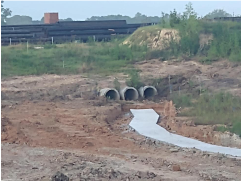
42" Outfall Pipe and channel at HS2 Detention Pond.
