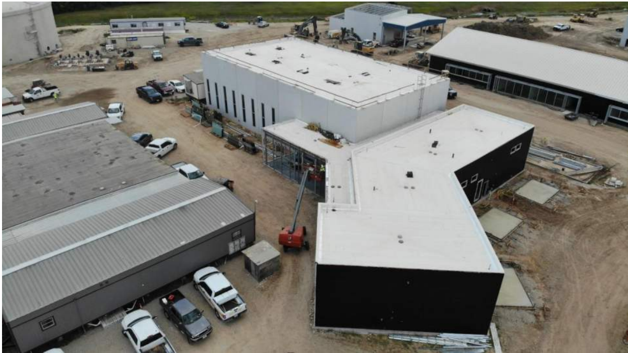
High Service Pump and Administration building. Note waterproofing and roof are complete
