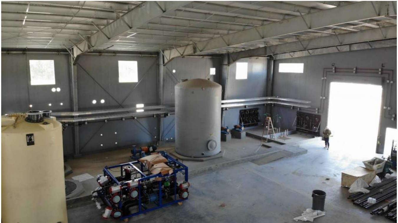
Process chemical storage equipment, pumps and tankage being set inside the membrane building
