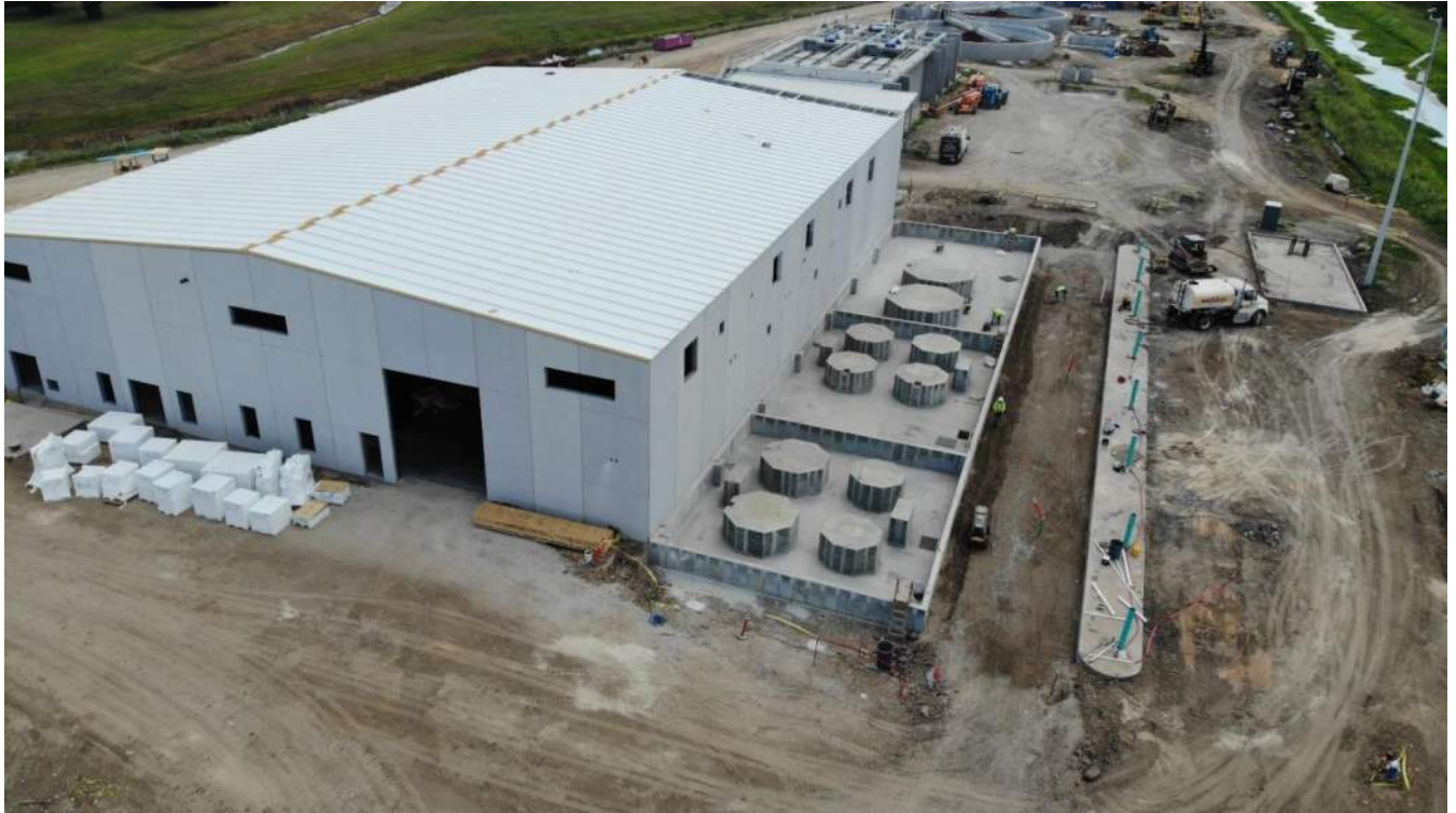
Membrane Building with bulk chemical storage area on close side. This storage area will be covered by a shed roof allowing deliveries to be brought in by truck and unloaded directly to the tank farm
