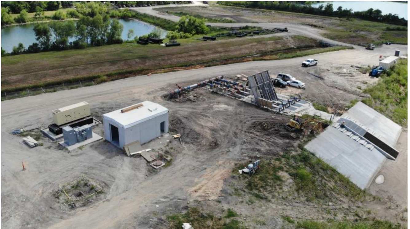
Raw Water Intake Lift Station and Electrical Building, note the vertical screens in the intake sump and the grated opening into the canal basin to the right.
