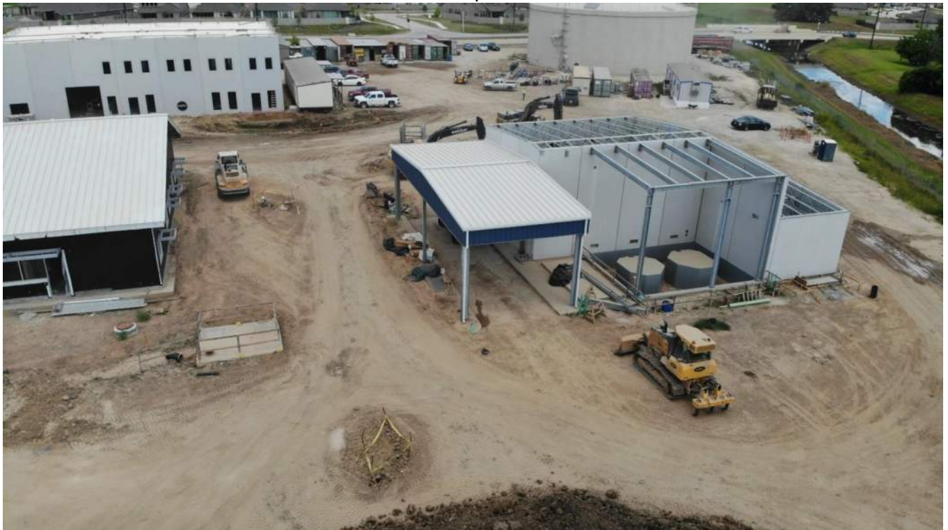
Chlorine Building will contain Chlorine gas cylinders, Chlorine Dioxide generator and Chlorine Scrubber
