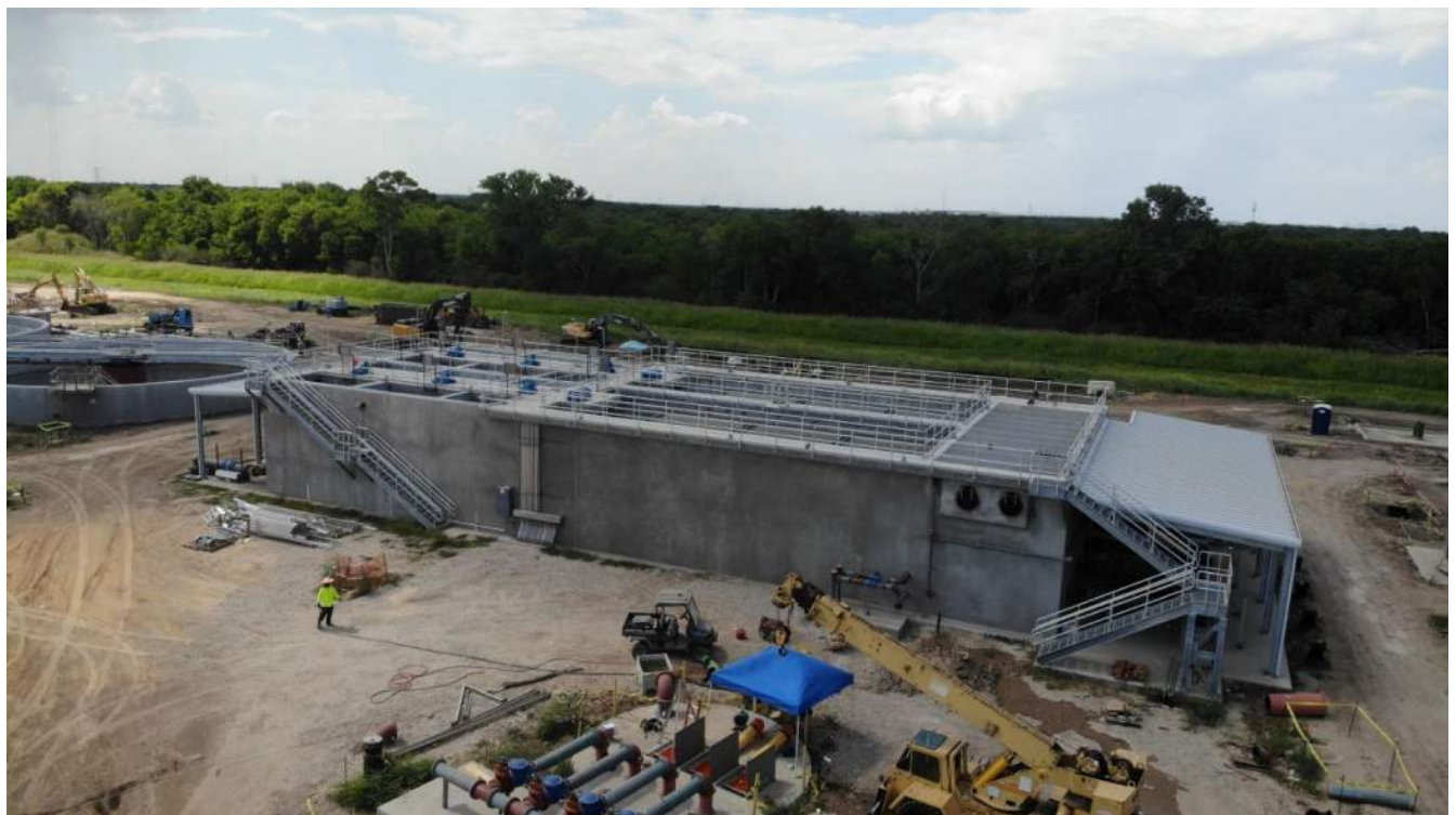
Pre-Treatment Basin nearing completion will be one of the first units to begin start-up following the Raw Water Intake Lift Station.
