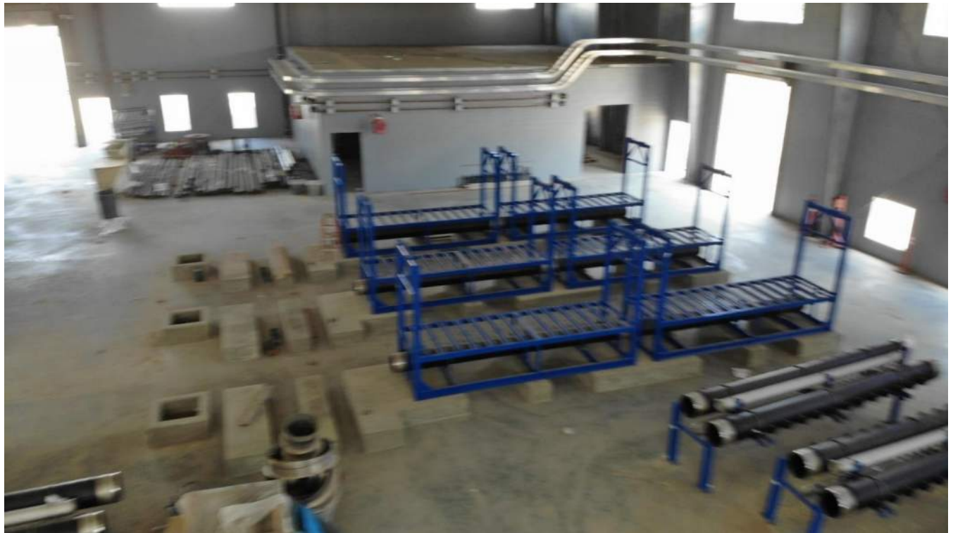
Membrane racks being installed inside the Membrane Building, note electrical and instrumentation raceways installed against the exterior walls.
