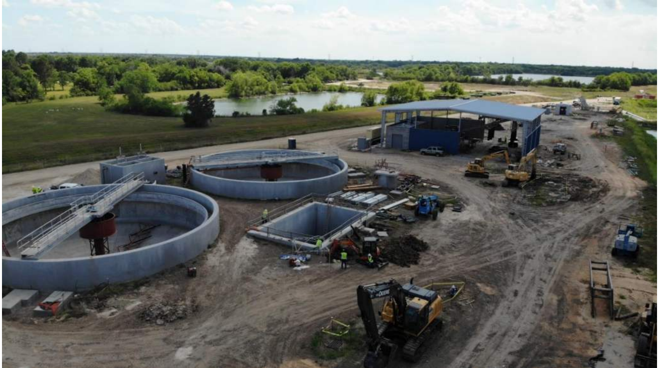
Solids Handling system consisting of Sludge Thickener, Washwater Recovery in the foreground and Belt Press DeWATERing facilities in the fare background.
