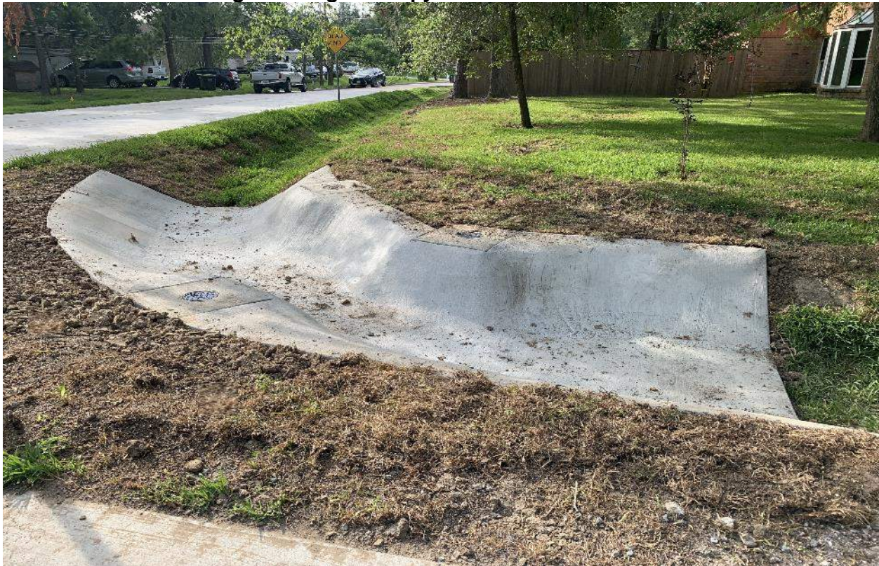
Slope Paving in Drainage Ditch at Sleepy Hollow and Rip Van Winkle
