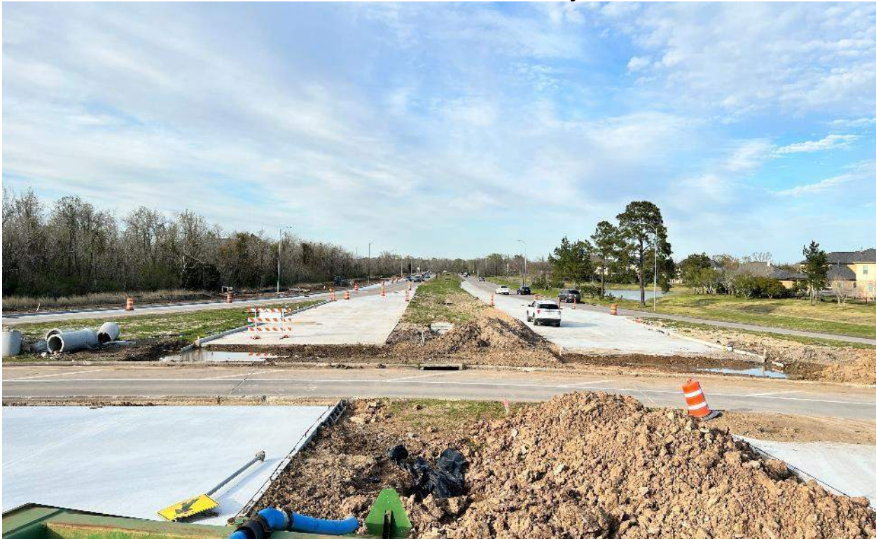
New Concrete Ready to be Tied into Each Other Once TCP is Implemented (North Side)
