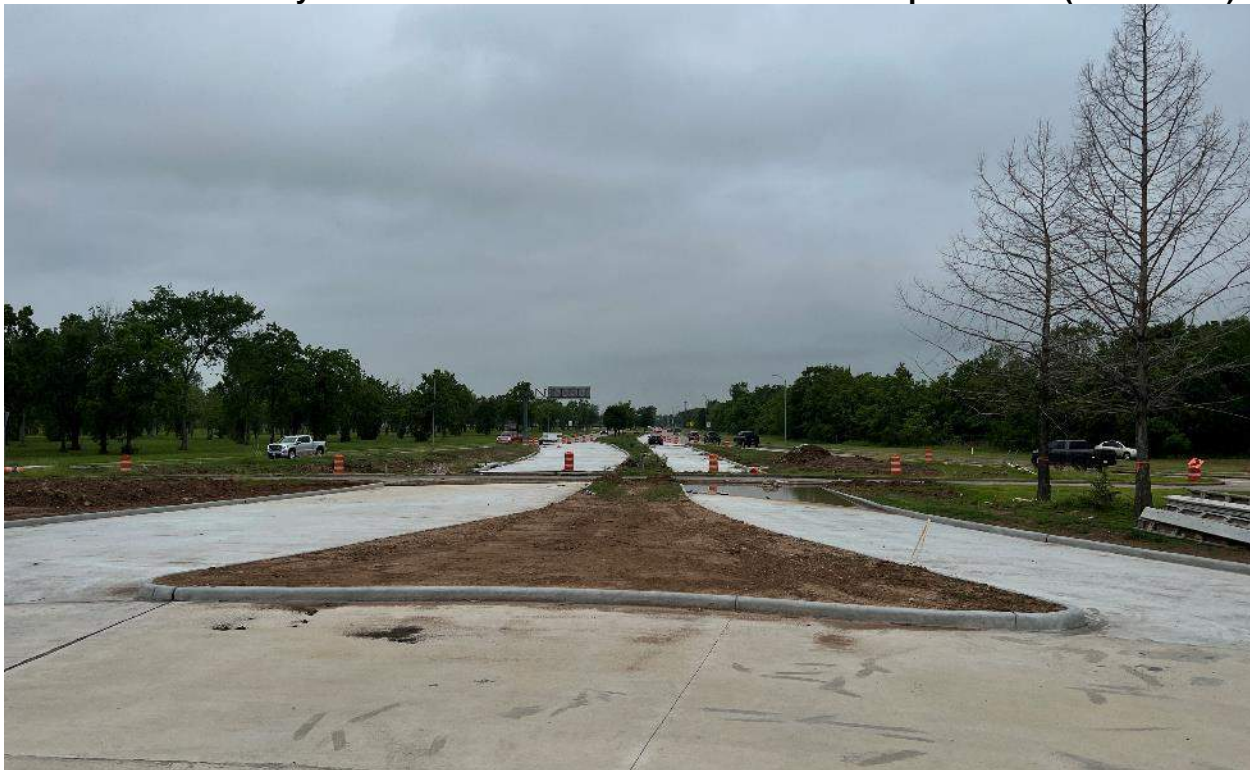
New Concrete Ready to be Tied into Each Other Once TCP is Implemented (West Side McHard)
