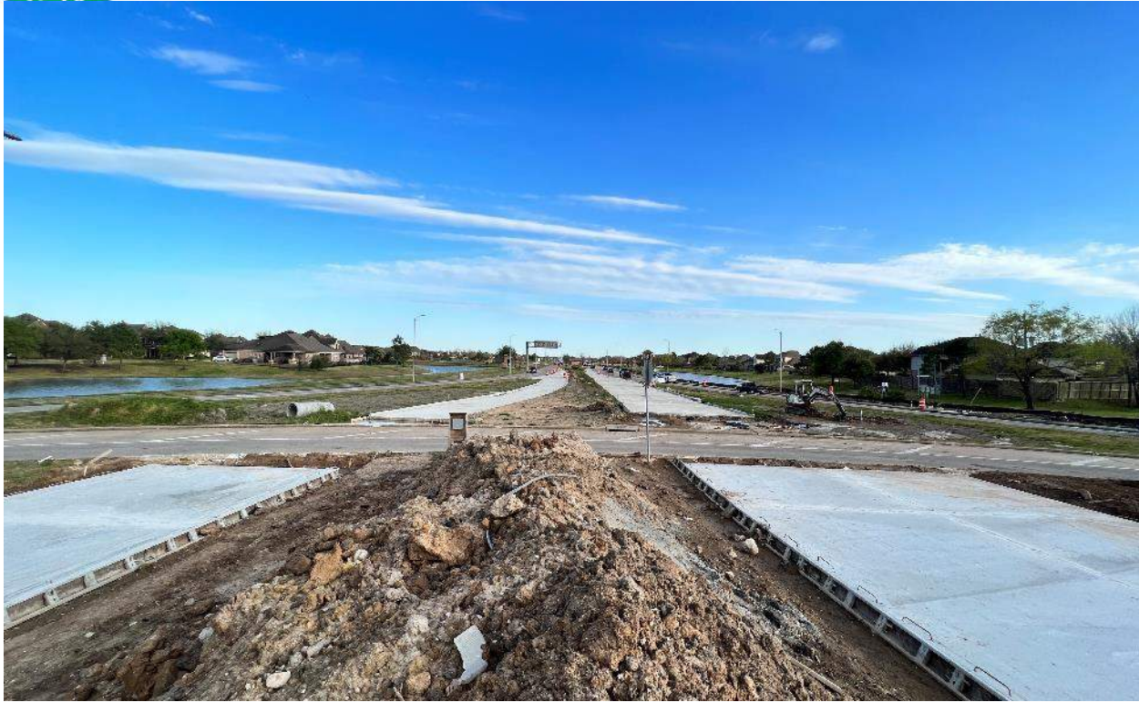
New Concrete Ready to be Tied into Each Other Once TCP is Implemented (South Side)
