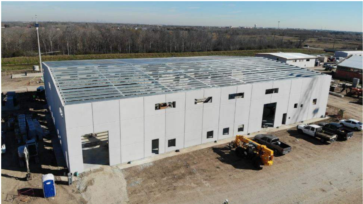
Membrane Bldg south wall showing roof and wall structure. This is the heart of the plant and must be capable of remaining in operation during storms. Precast concrete panel walls and reinforced roof provide that required level of storm resistance.
