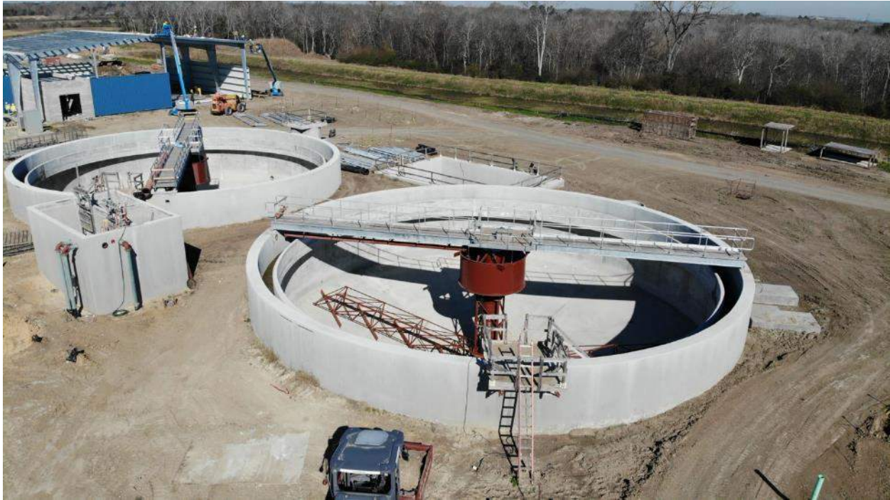
Gravity Thickener in foreground and Washwater Recycle in the background. The small structure in between these is the Belt Press Feed Pump Station. These structures were the first to be built on site avoiding the need to shore or bench the deep excavations.
