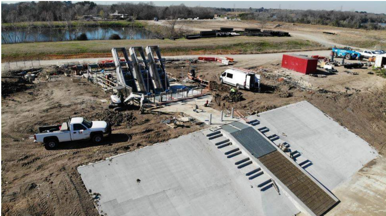
Raw Water Intake in canal bank with primary trash screens mounted above and below the ordinary water level in the canal. This allows the intake to continue to work during anticipated low water levels in the canal.
