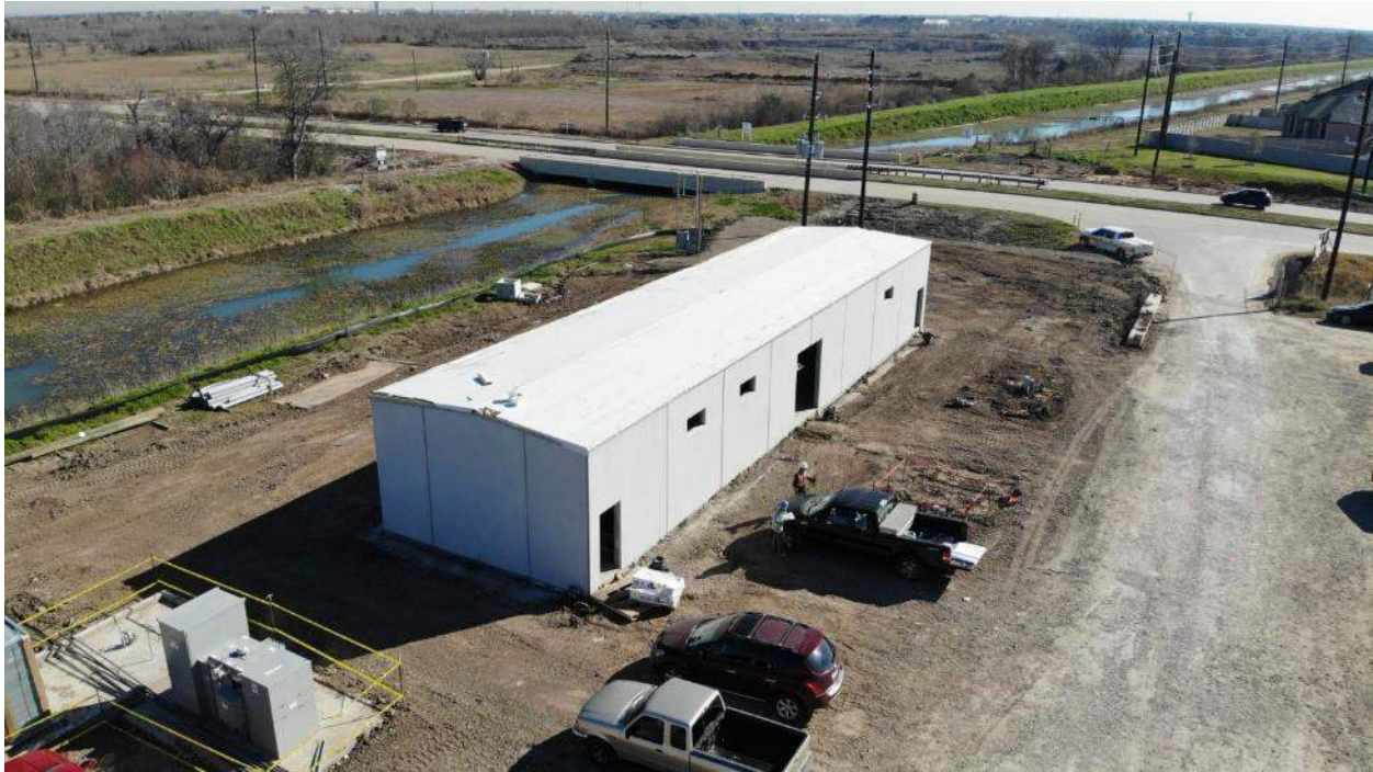
Main Electrical Building, West looking East, Location of the main gate in background and Permanent power entrance into the plant just beyond the Electrical Building
