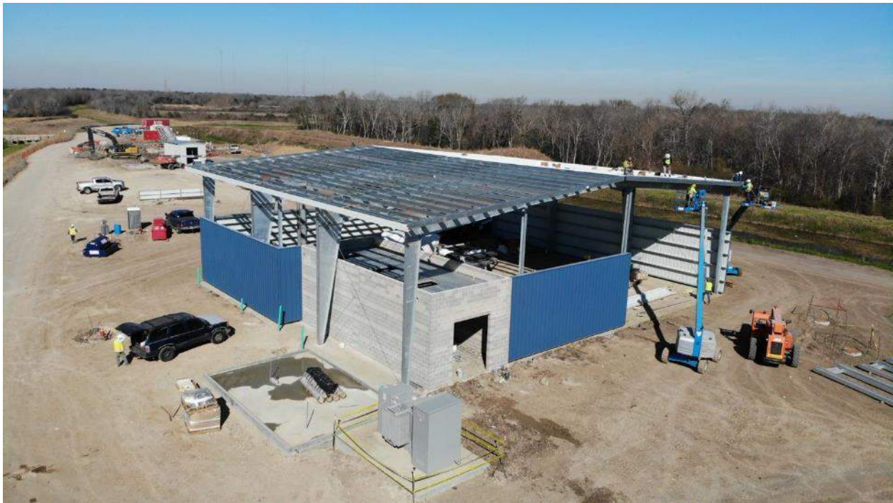
Solids Handling Bldg contains the Belt Presses and polymer storage and will house the solids transfer and truck loading operations. The loading bay is located towards the right hand side of the building.
