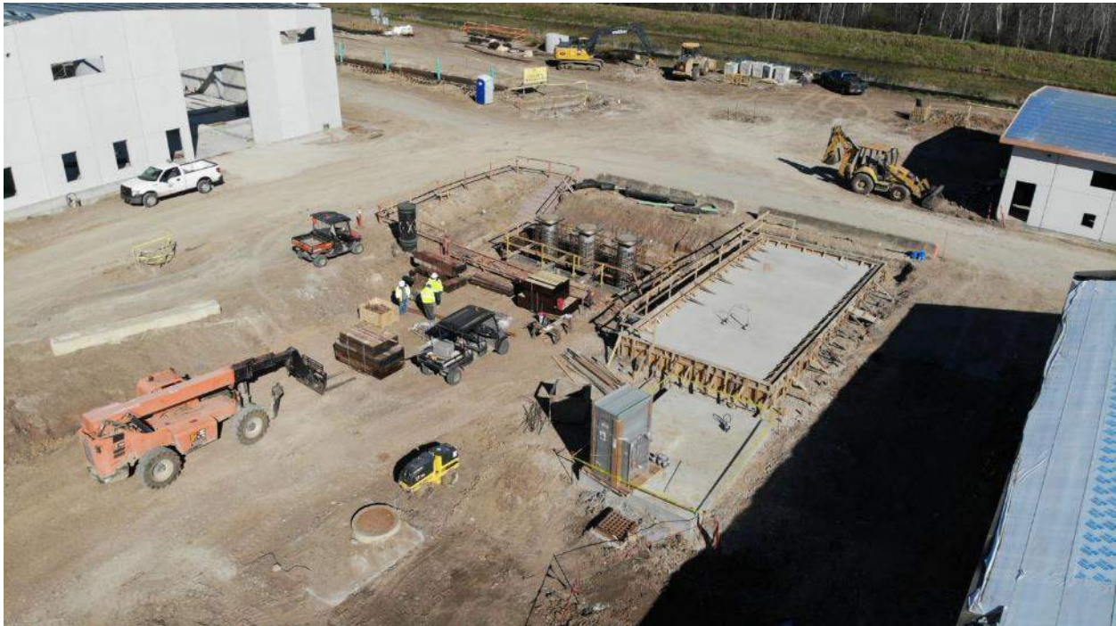
GAC Reactors Foundation and Chlorine Contact Transfer Pump Piping
