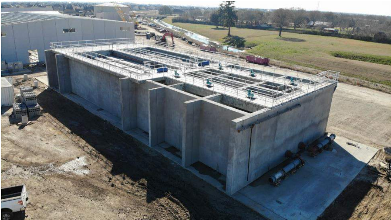
West end of Pre-Treatment basin showing Raw Water intake piping
