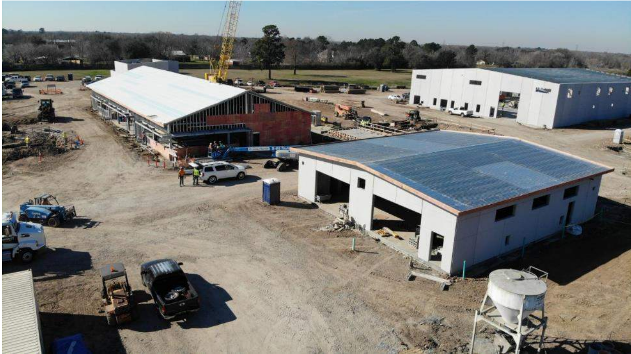
Maintenance Bldg in foreground Operations Bldg and Membrane buildings behind
