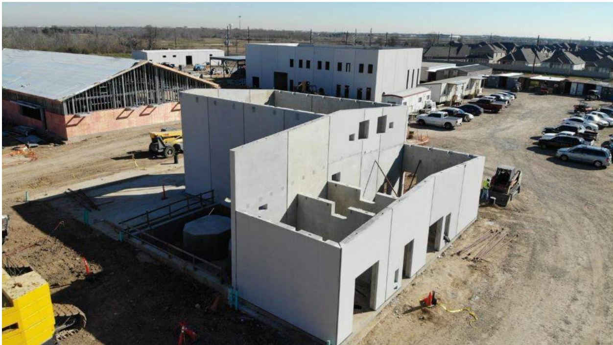
Back side of the Gas Chloring bld'g showing (front to back) Electrical Room, Mechanical Room and Chloring Generator Room with outdoor storage area to the left front and Chlorine gas storage room left rear.
