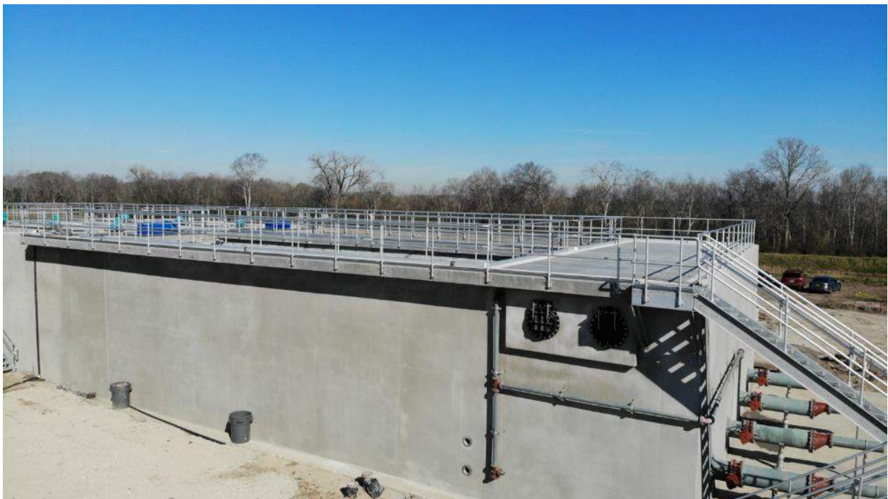
South side of Pre-Treatment Basin showing completed installation of the over-flow flapper gates to the right below the catwalk.
