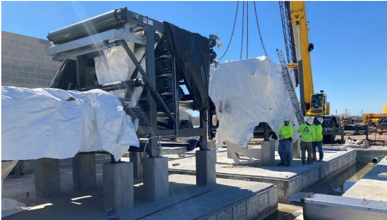
Belt Presses were set, shimmed and bolted down in mid-February prior to the installation of the building structure.
