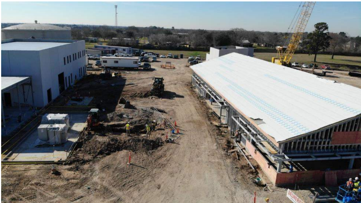
Front view of Operations Bldg from South end with High Service Pump and visitor Center on left
