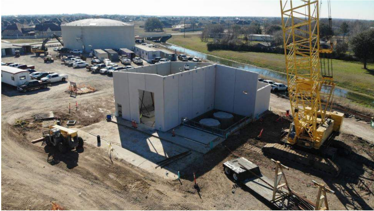
Gas Chloring and Chlorine DiOxide bldg. pre-cast exterior wall panels being erected.
