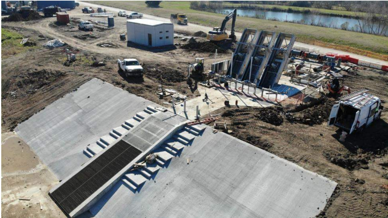
Raw Water intake and slope paving on canal bank. Note the cast in stair steps for maintenance access to the primary screens. Lowest step is below the ordinary normal water elevation of the canal.
