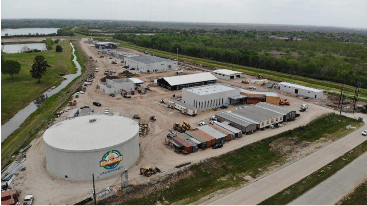
Overall Site View from southeast. Note CMAR's temporary offices and material storage that will be removed to complete installation of finished water transmission line and Plant Service Water ring. CMAR & City Staff will move into Admin and Operations for this installation.
