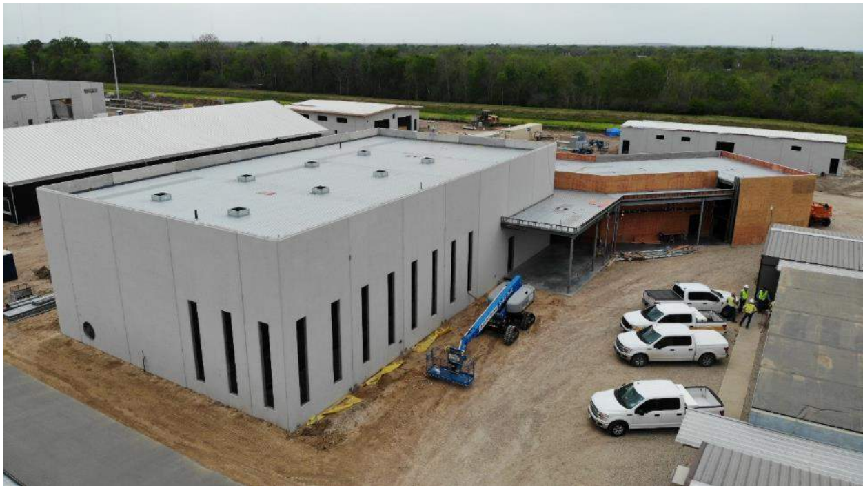
Front of the High Service Pump Bldg. public's view of the plant
