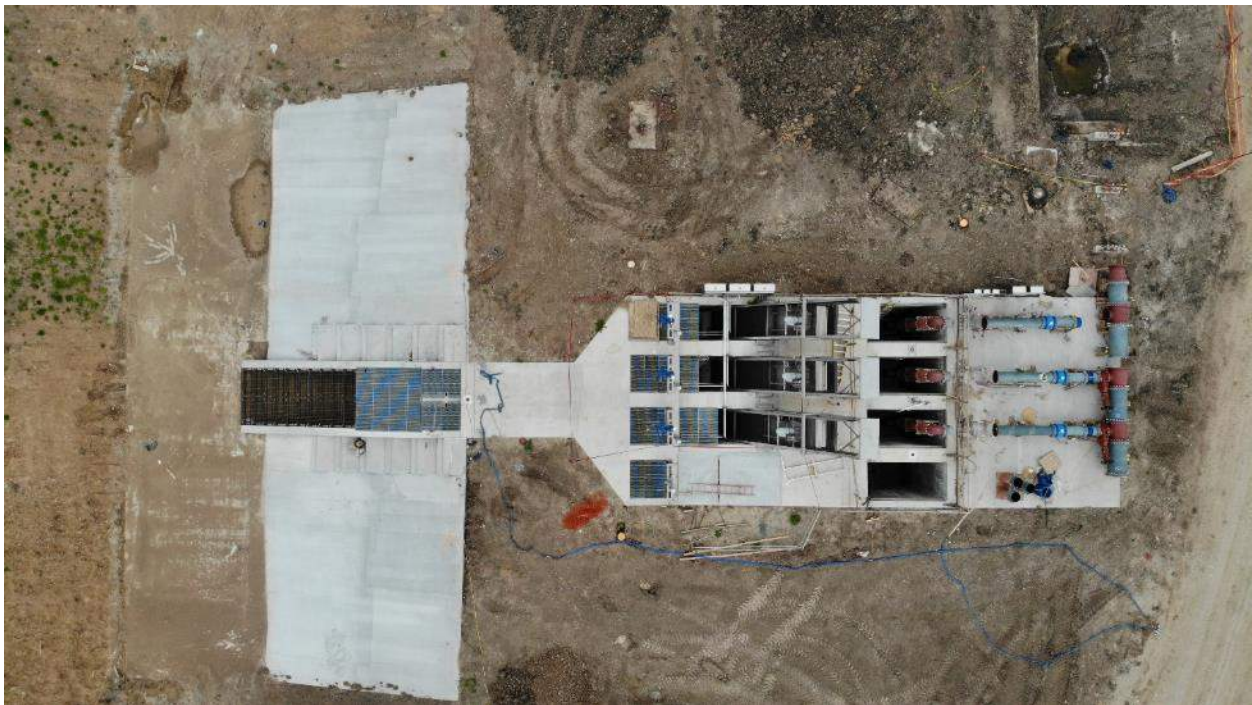
Direct overhead view of Raw Water Lift Station showing Debris Vertical Rakes and pump wells
