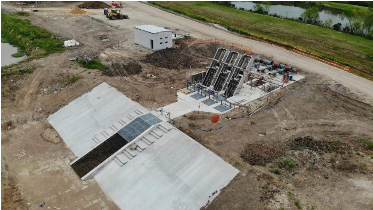
Raw Water Lift Station and Canal Bank slope paving with debris strainer
