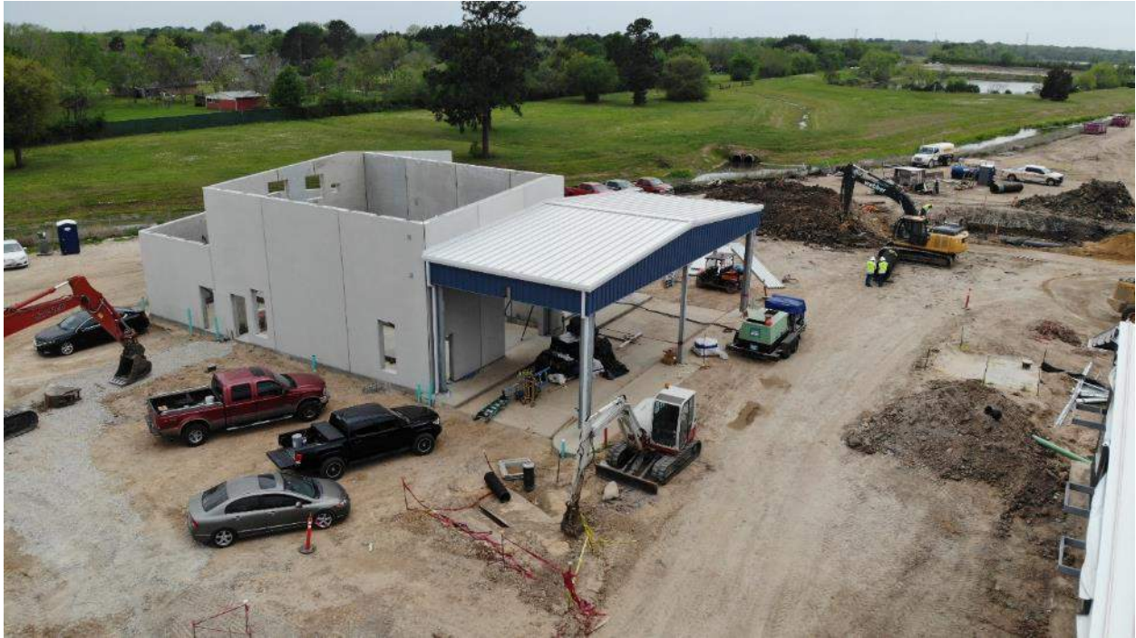
Chlorine DiOxide Bldg.
