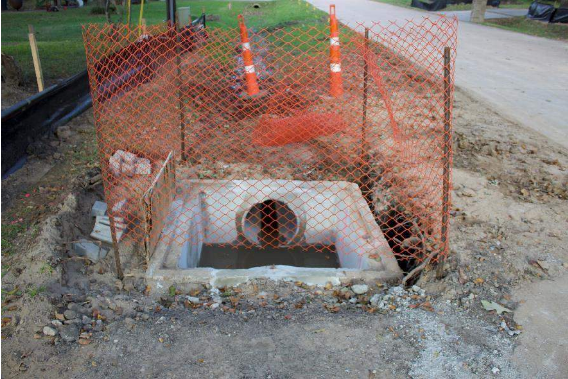
Storm Inlet Box Have Been Set in Place and Culverts Have Been Grouted In
