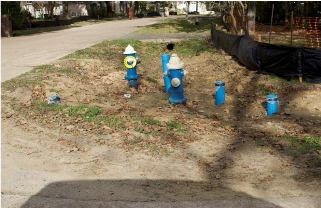
New Fire Hydrant Assemblies and Valves Have Been Installed, old one will be removed once the new line is fully operational
