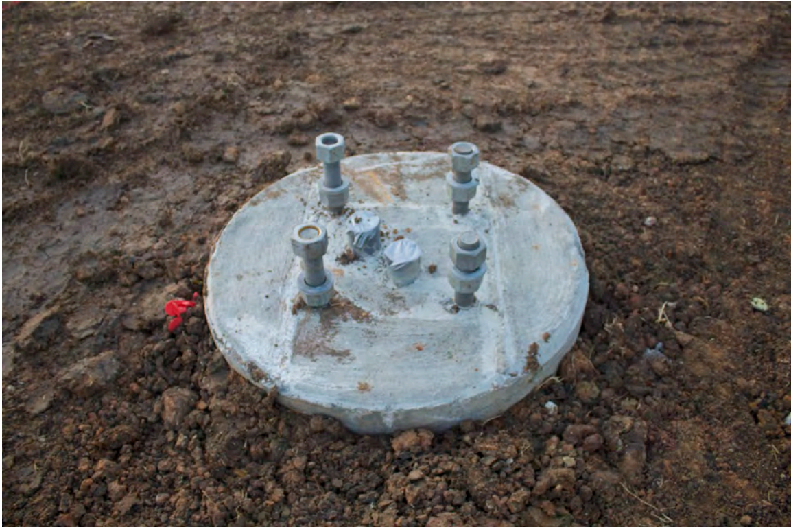
Traffic Signal Bases have been Poured at Forest Park and Pearland Parkway
