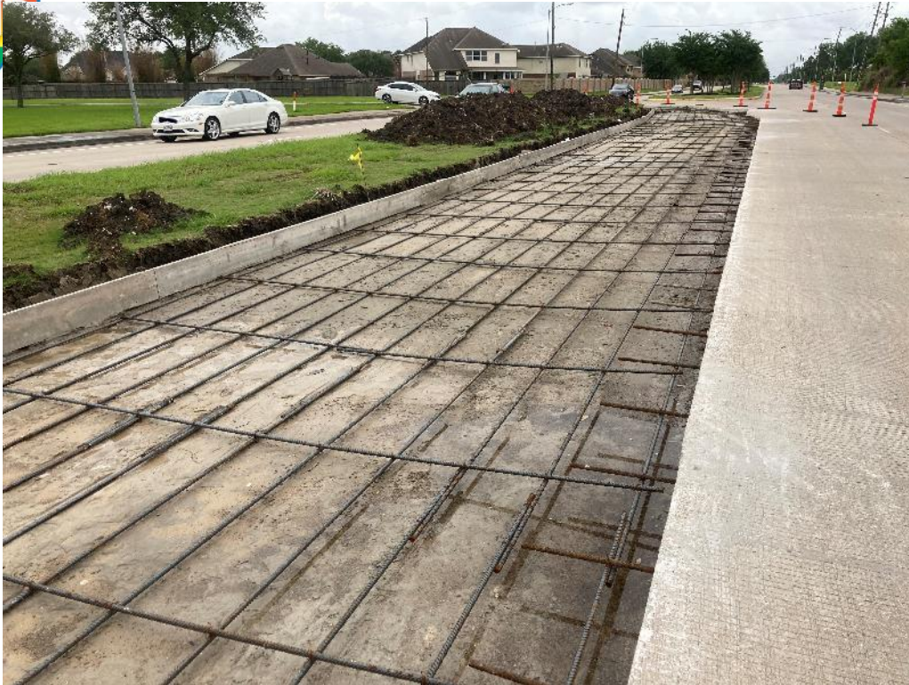
Left Turn Lane Formed and Rebar is Tied at Dixie Farm Road and Long Oak Dr.
