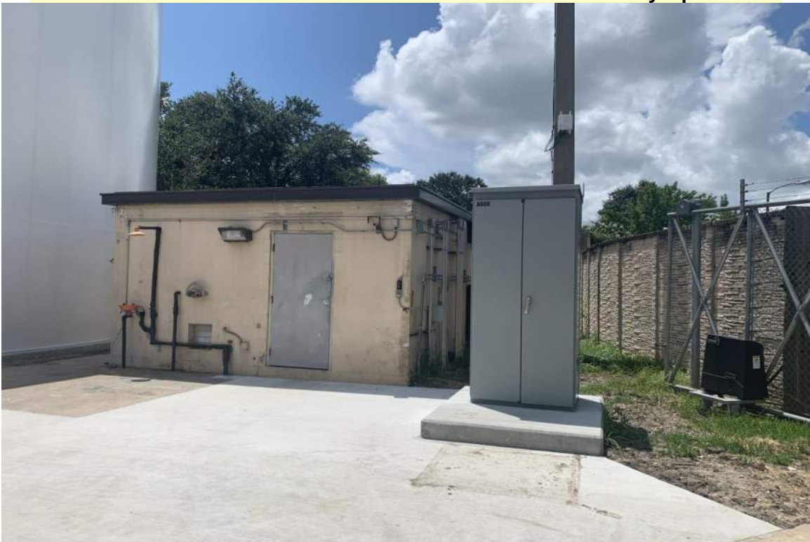
Generators Automatic Transfer Switch
