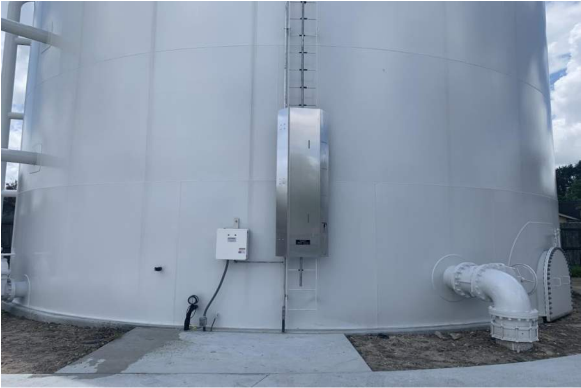
Exterior Ladder Anti-Climb Cage Installed and Secured
