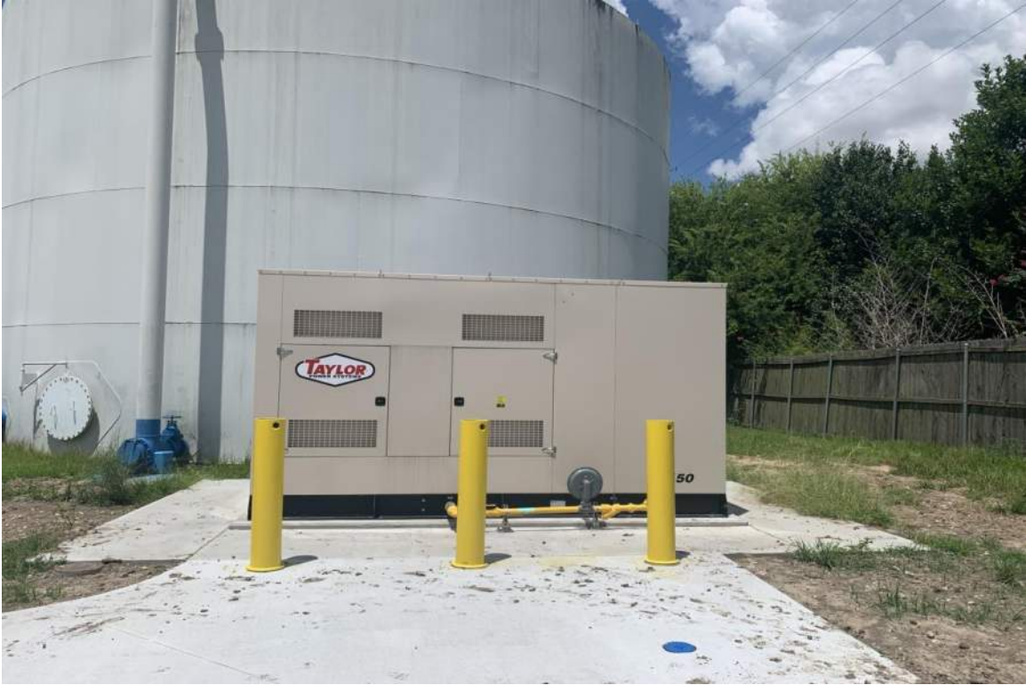
Gas Service to Generator has been Established and Unit is Fully Operational
