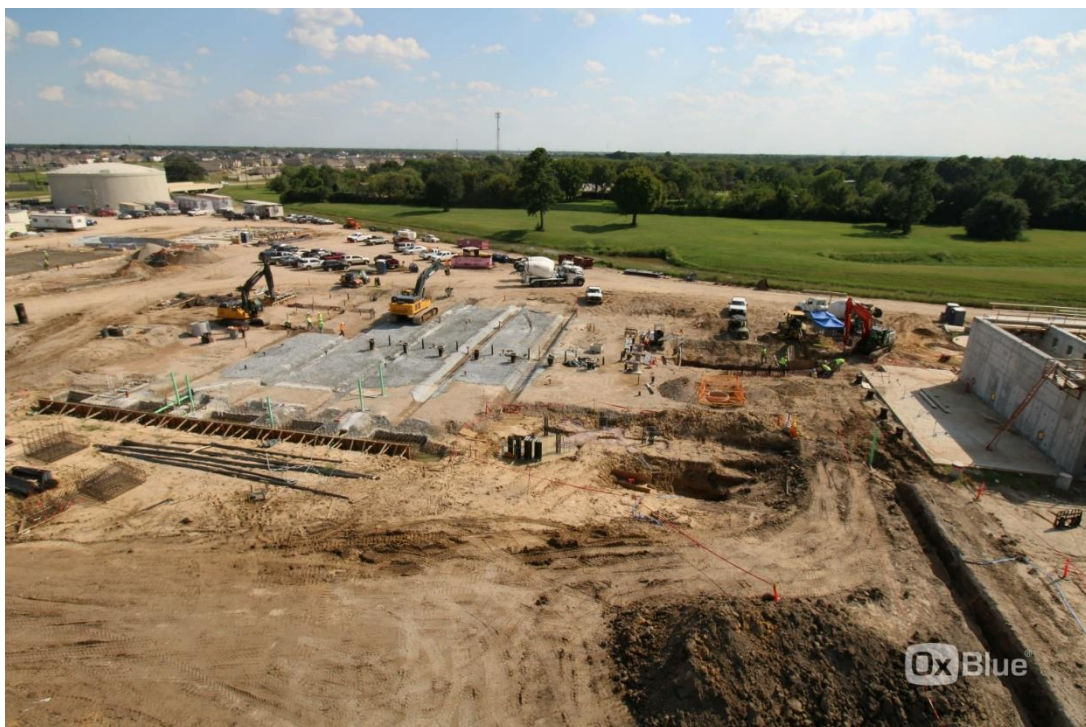
View of the Membrane Building foundation and below grade piping
