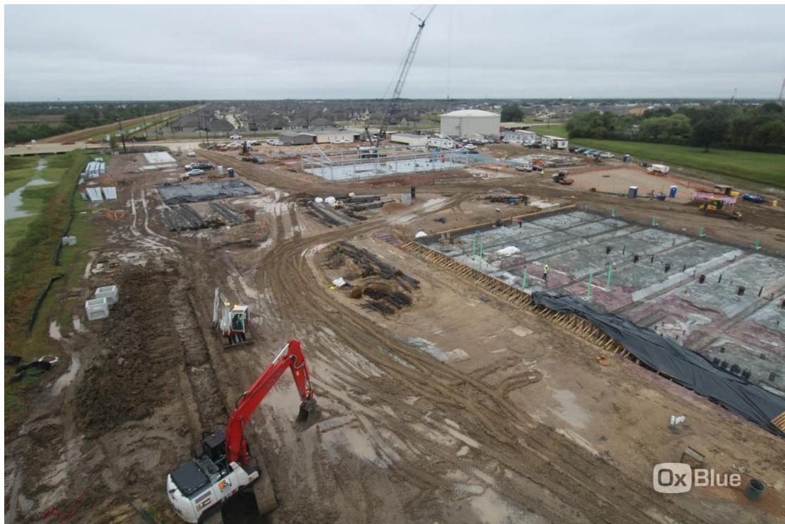
View looking east/ Southeast with the membrane building foundation preparations in the foreground and the Operations building structure being assembled in the background
