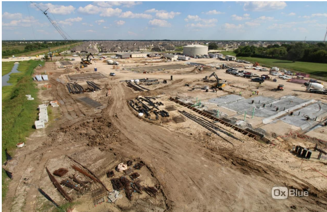
Looking East; Membrane Building foundation in foreground with Operations Building foundation immediately east, maintenance Building to the north (left) and Electrical Building foundation just beyond the crane.
