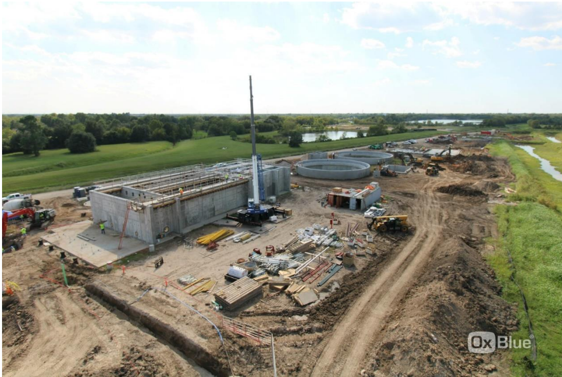
Site view looking West showing Pre-Treatment Basin in the foreground with Gravity Thickener and Wash Water Recovery facilities immediately west. In far background is the foundation for the Solids Processing/ Belt Press Filter building
