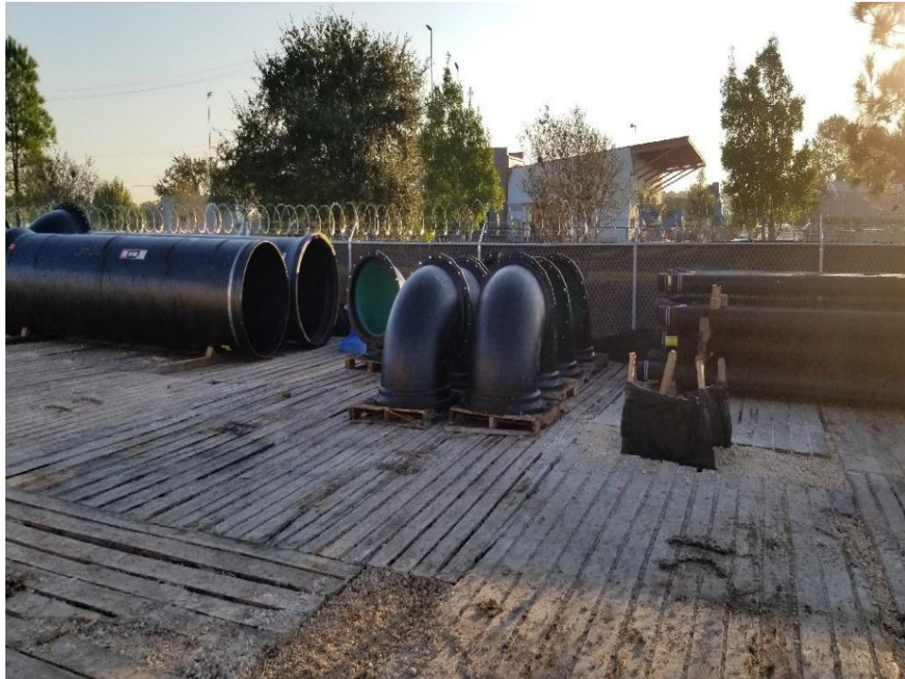
30" and 48" ductile iron pipe on the east side of the plant.
