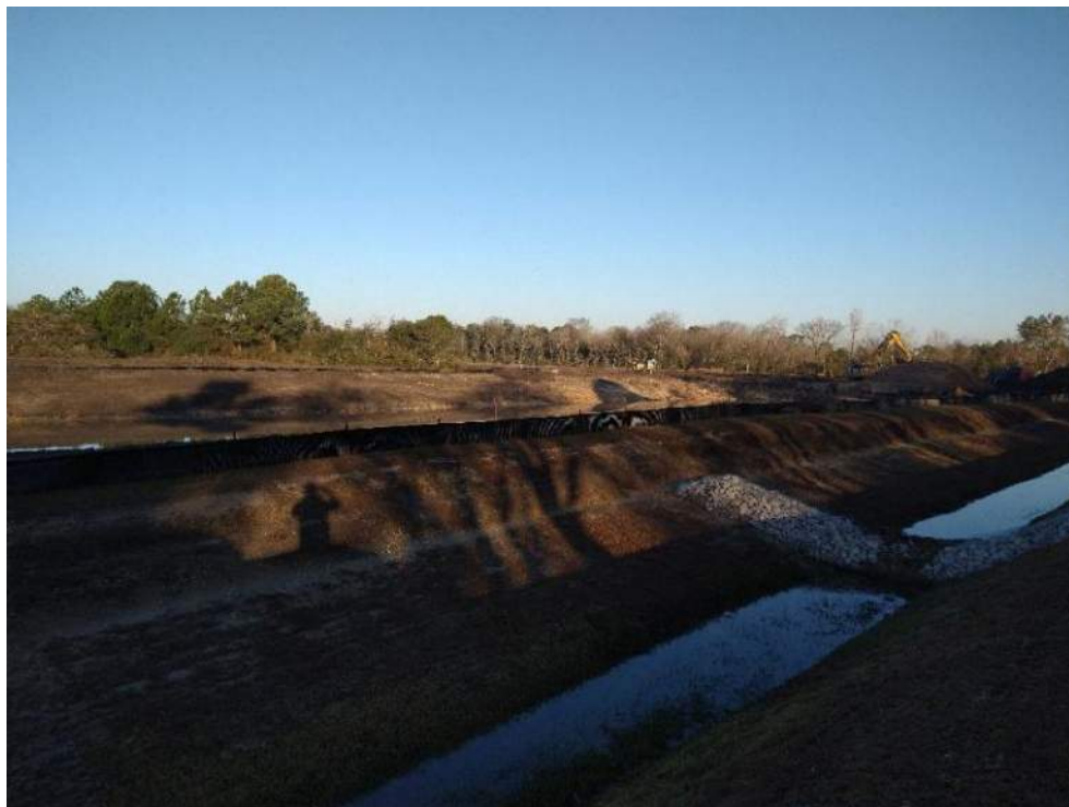
Hickory Slough Drainage System Detention Pond 1
