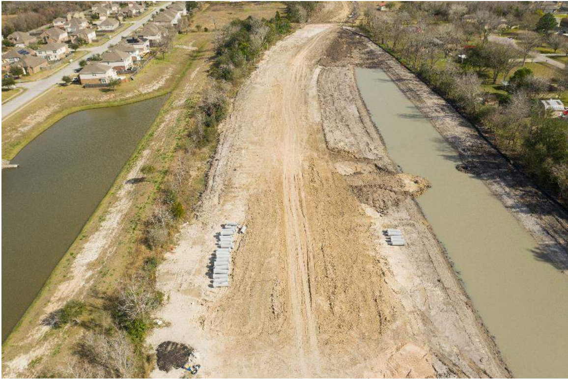
Hickory Slough Drainage System Detention Pond 1
