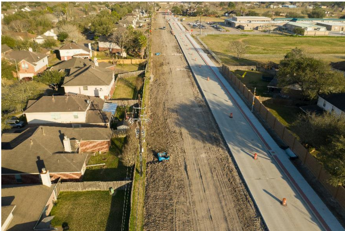
Long range shot showing completed lanes & sidewalk with Challenger Elementary in the right side background
