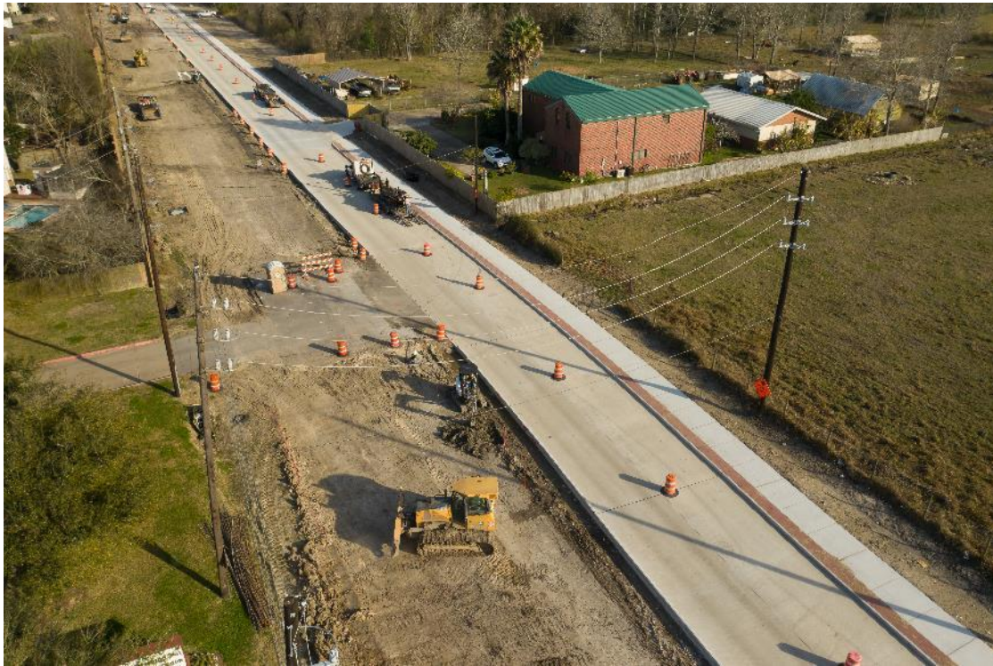
East end of project showing completed E-bound lanes with Sidewalk & Paver strip
