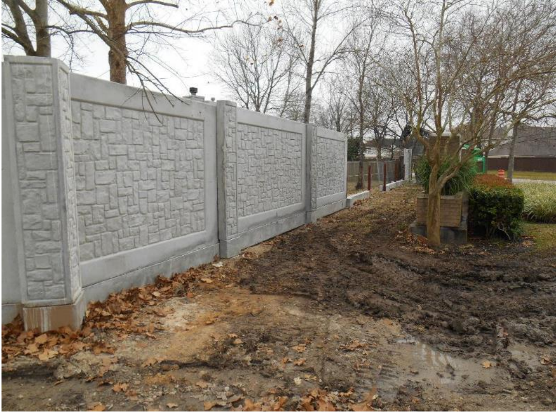
Unpainted Sound Wall installed near Miller Ranch Intersection
