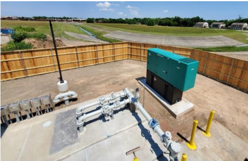
Package 2 - Orange/ Mykawa New Generator
