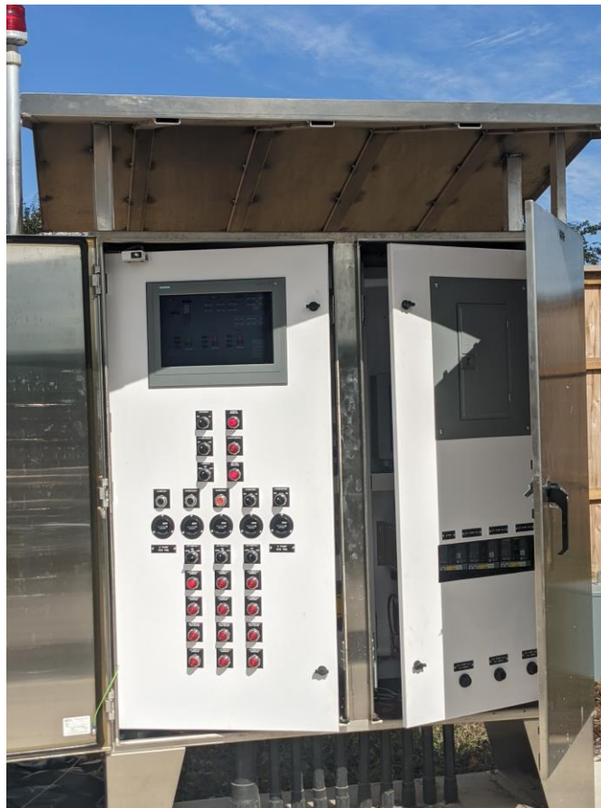
Package 2 – New Electrical Control Panel at Orange/Mykawa LS
