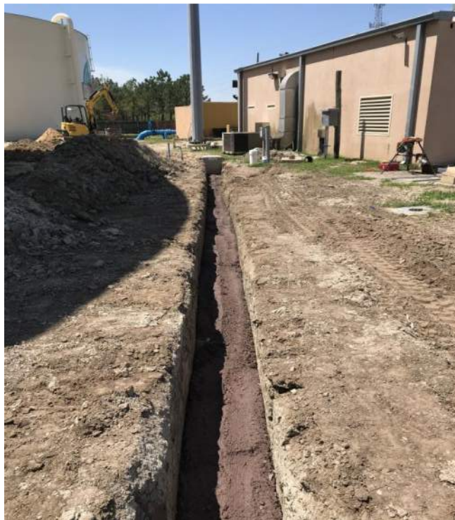
Red concrete ductbank
