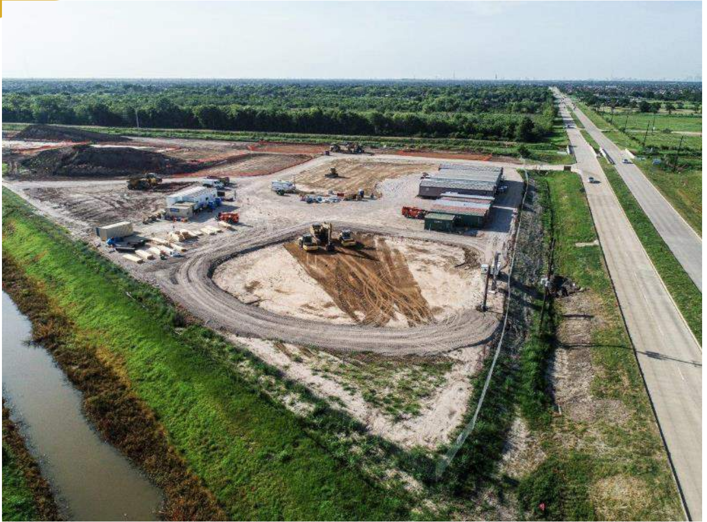
View from Southeast corner showing GST soil foundation in forefront. Behind and further north in the foundation for the High Service Pump building and west of that is the foundation for the Operations control building.
