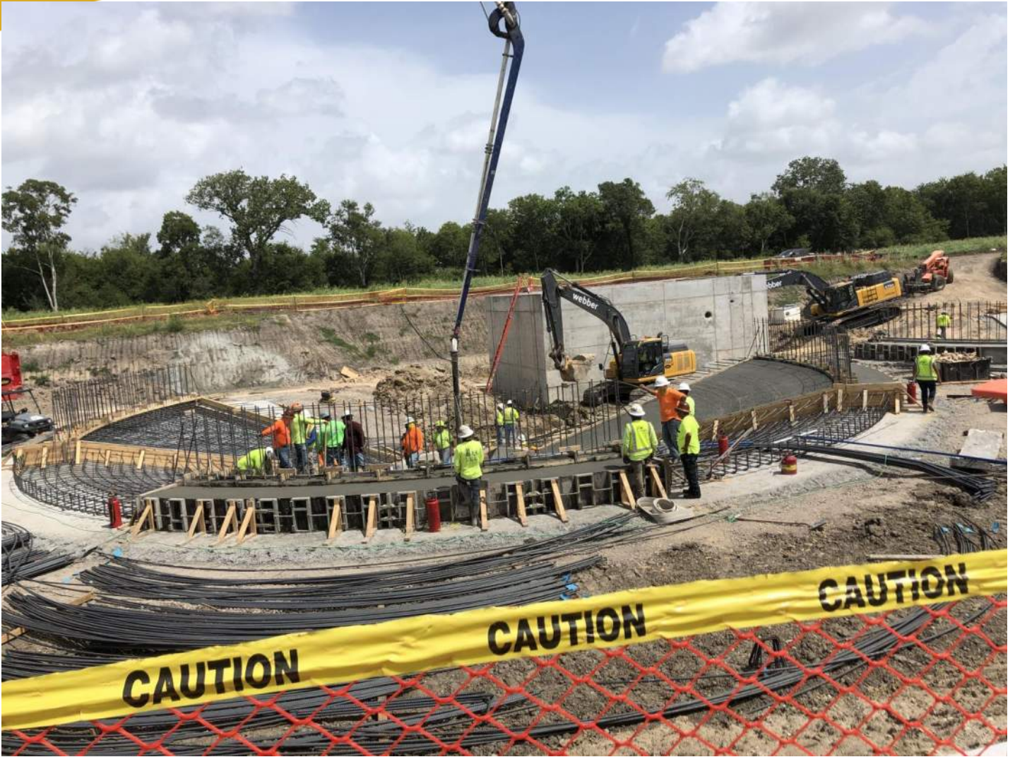
This photo was taken at the end of August showing concrete formwork and reinforcing for the concrete floor of the Gravity Sludge Thickener with the Belt Press Pump basin in the background.
