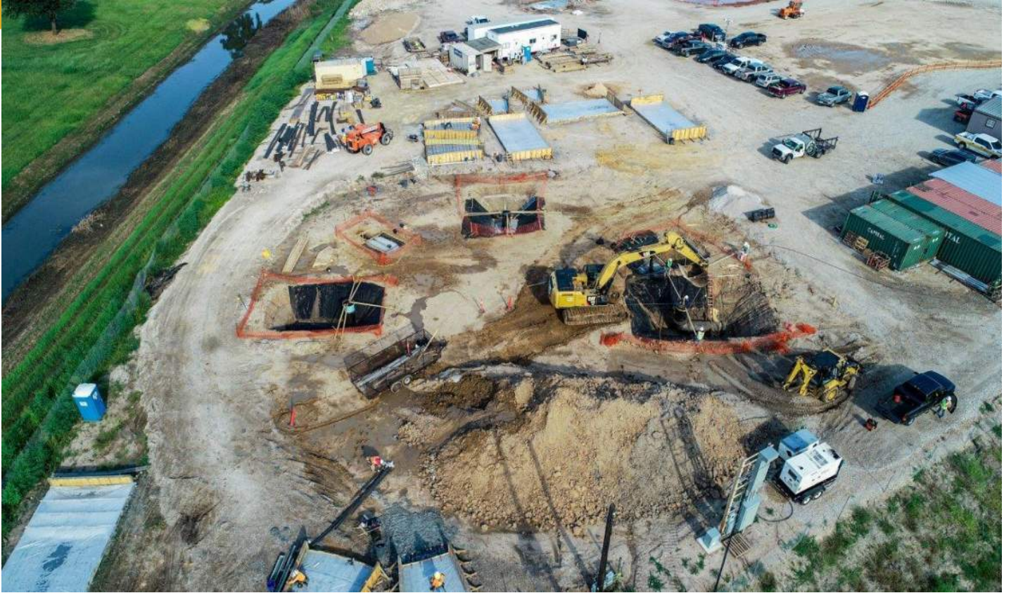
This shows the soil foundation for the GST with casting beds for tank wall and roof panels and installation of under-floor drain piping being installed by the tank sub-contractor DN Tanks.
