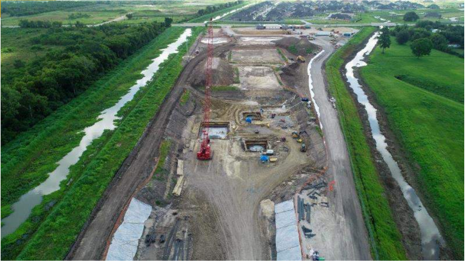
Mustang Bayou on right and GCWA source water canal on left. Foreground shows foundations for De-Watering and Belt Press Filter building with Sludge Thickeners, and BFP Pump Basin in the center. Further east is the Pre-treatment facility foundation followed immediately by the membrane building foundation. This photo was taken during the heavy rains at the end of July.
