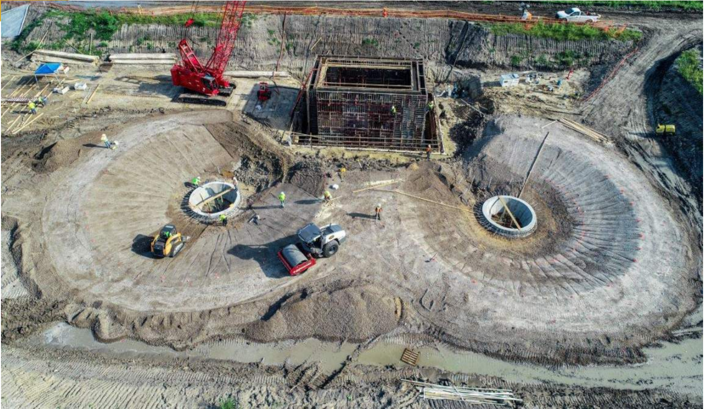
This is the same Gravity Sludge Thickeners and BFP Pump Basin approximately two weeks later showing progression of the work. This photo was taken about two weeks later, mid-August showing extensive soil foundation work going in around the preliminary concrete.
