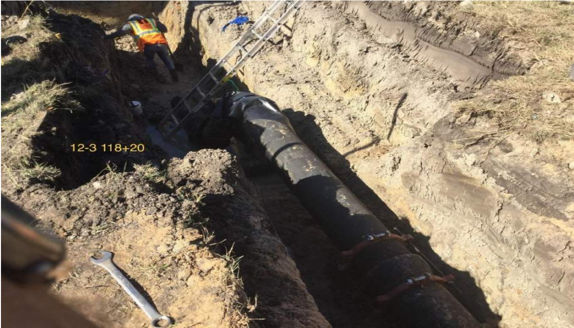
Recently bored 16" water line in 24" steel casing at O'day/ McHard Road Intersection.
