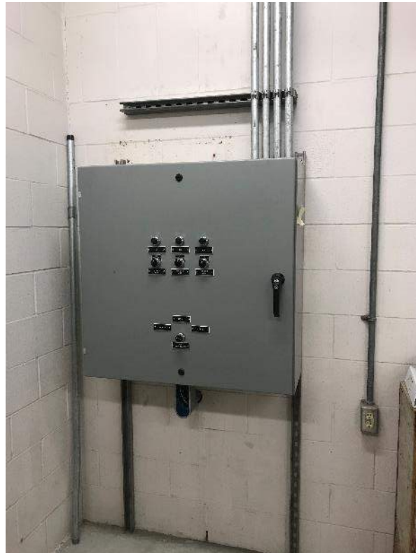
New control panel for the tank
