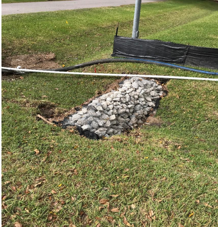
SWPPP Rock Dam
