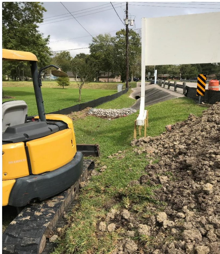
SWPPP Rock Dam
