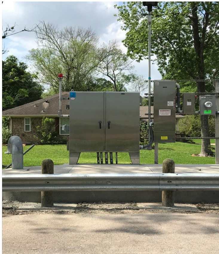
New Lift Station
