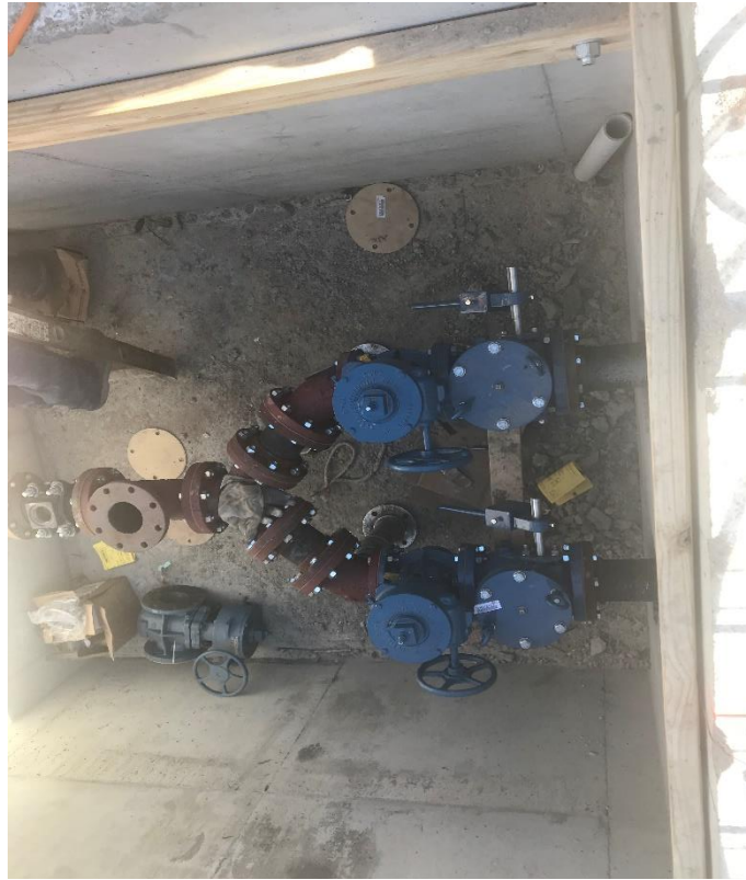
Valves and pipes in vault
