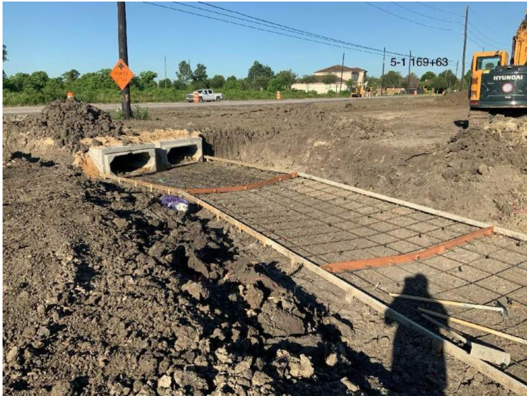
Storm sewer System C outfall into Detention Pond X with slope paving formed up.
