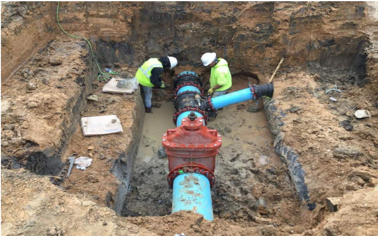
16" x 8" Wet connection located near the Bailey Road Water Treatment Plant.
