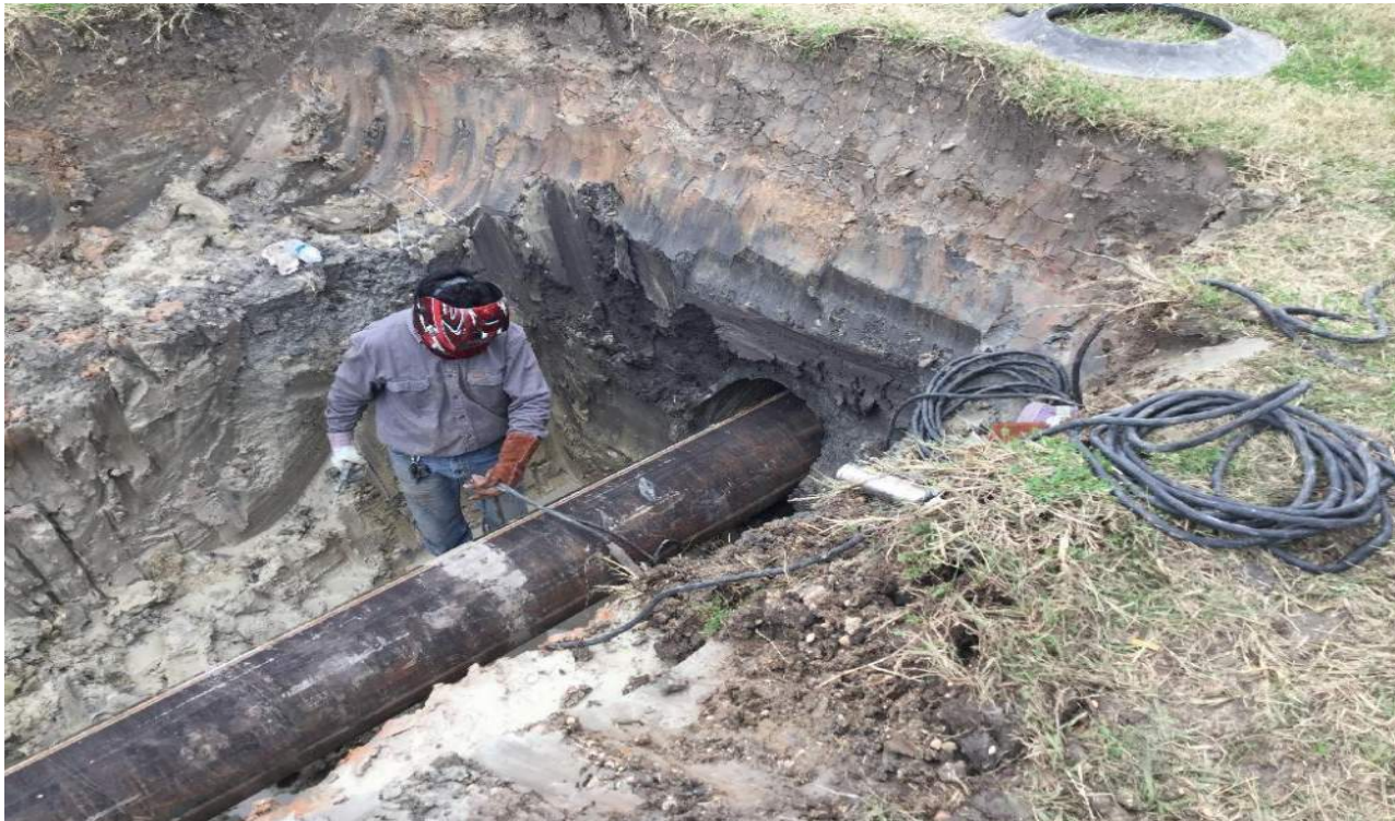
Welder in the trench welding segments of casing as it gets pushed through the bore hole.
