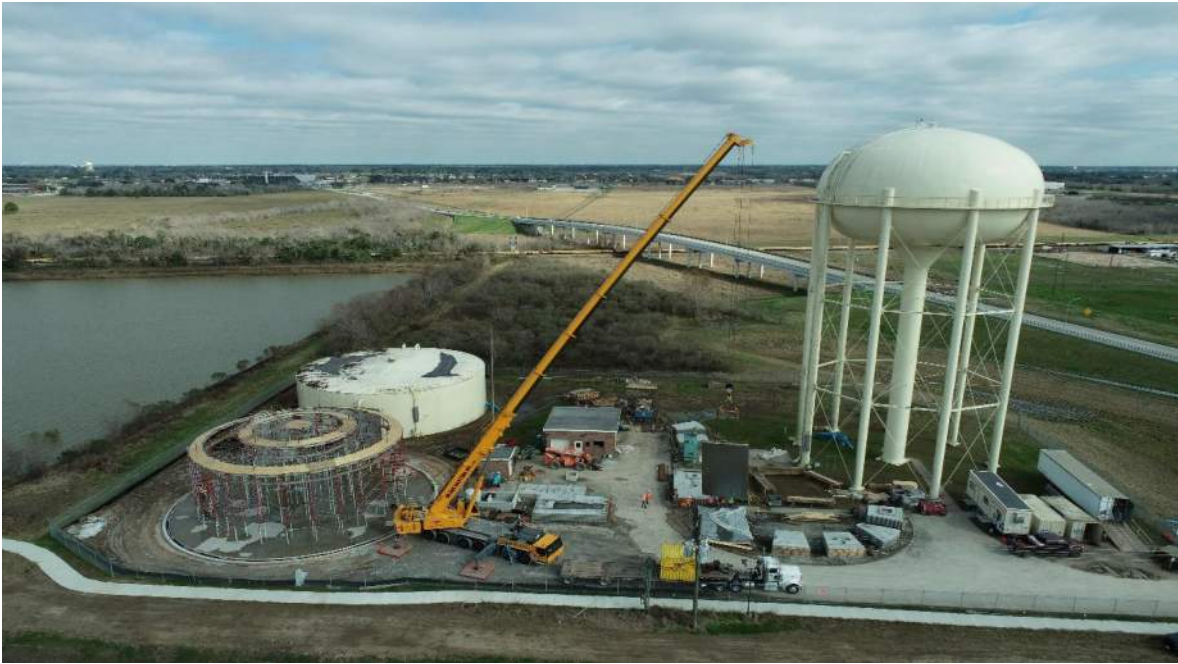
Aerial view of the ground storage tank (GST). Wall panel in motion to be installed
