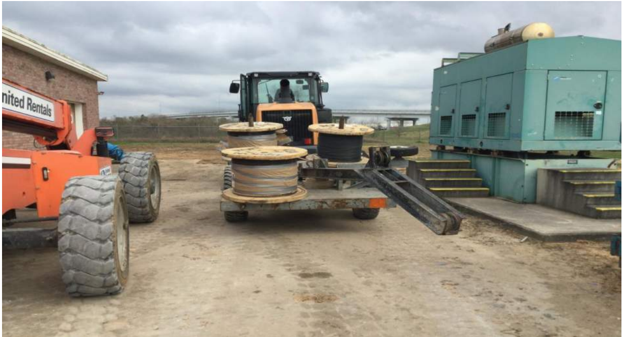
Winding equipment that will be used to run pre-stress cable around GST.
