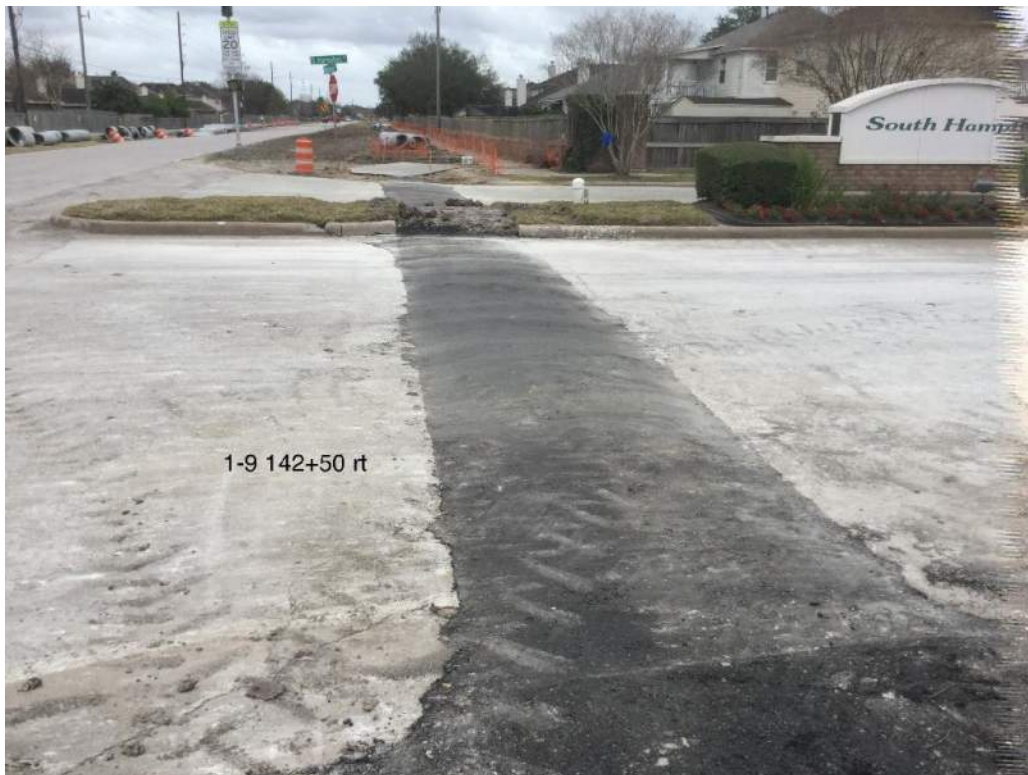
Storm sewer crossing at South Hampton, temporary patch. 01-09-2020
