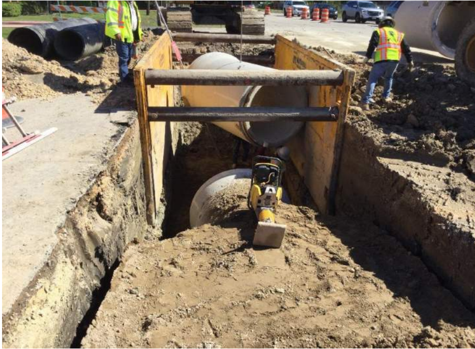
Installing storm sewer at the intersection of Hughes Ranch Rd/Smith Ranch Rd. 10-30-2019
