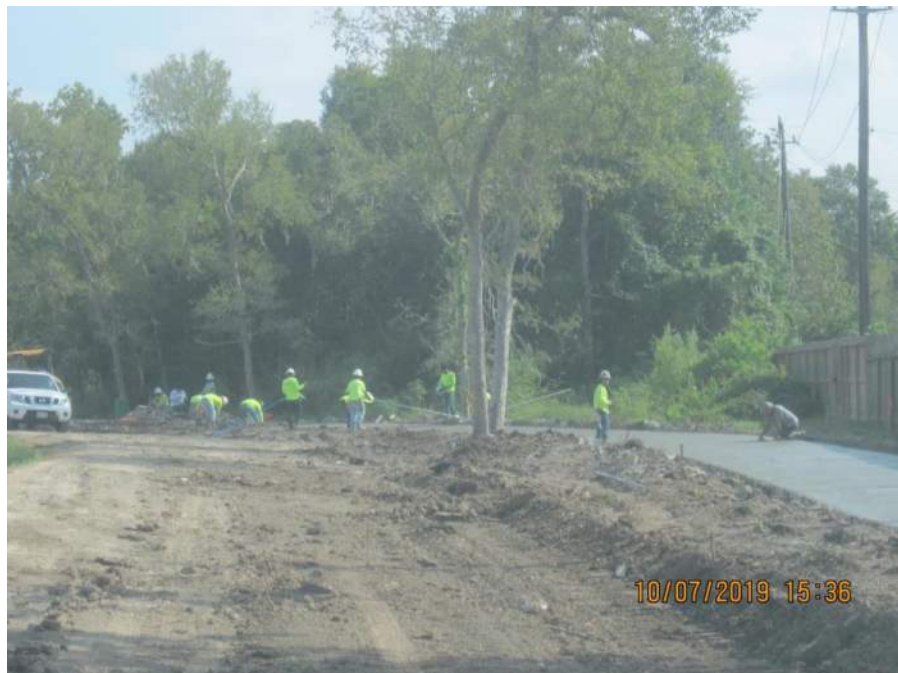
Brazoria County Portion of Trail, concrete pour behind Clear Creek Park Subdivision.
