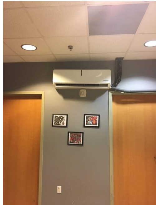
Secondary Air Conditioner Units
