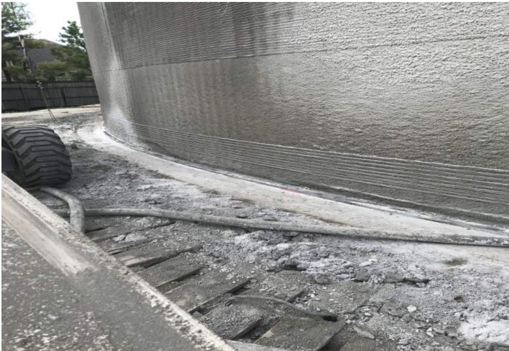
Building forms to pour curb inside tank to connect slab to the walls.
