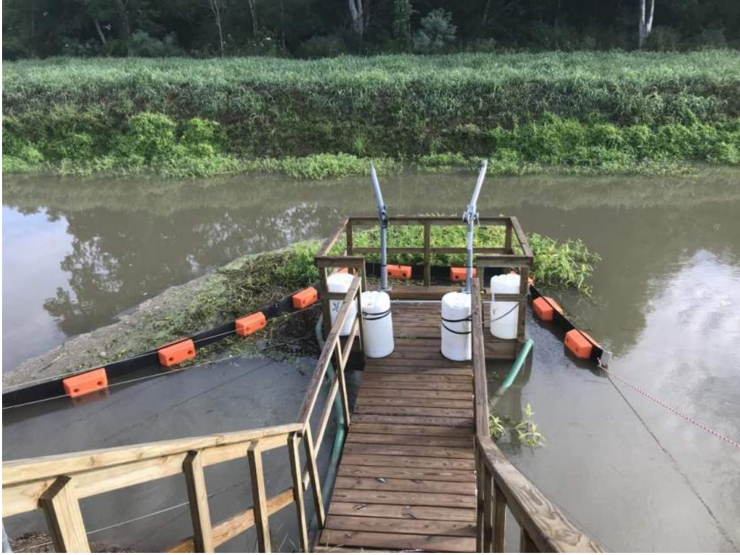
Raw Water Intake Pumps
