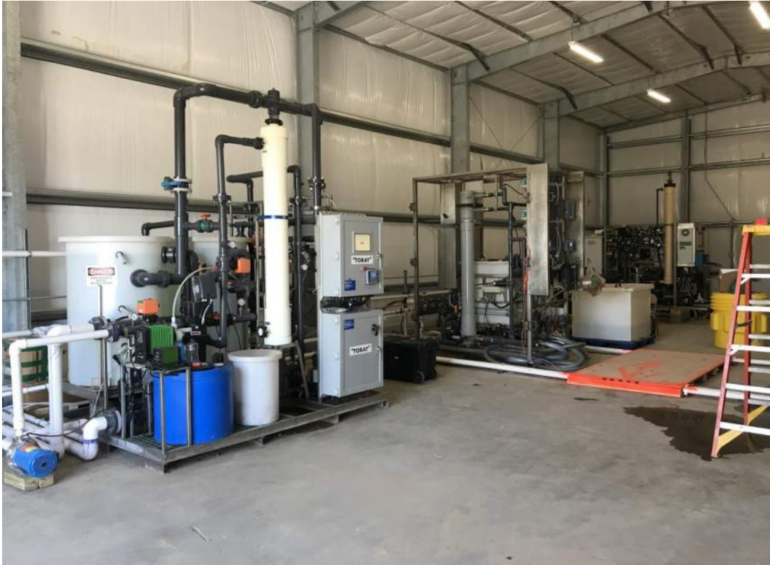
Membrane Filter Units - Toray, Evoqua, and Pall
