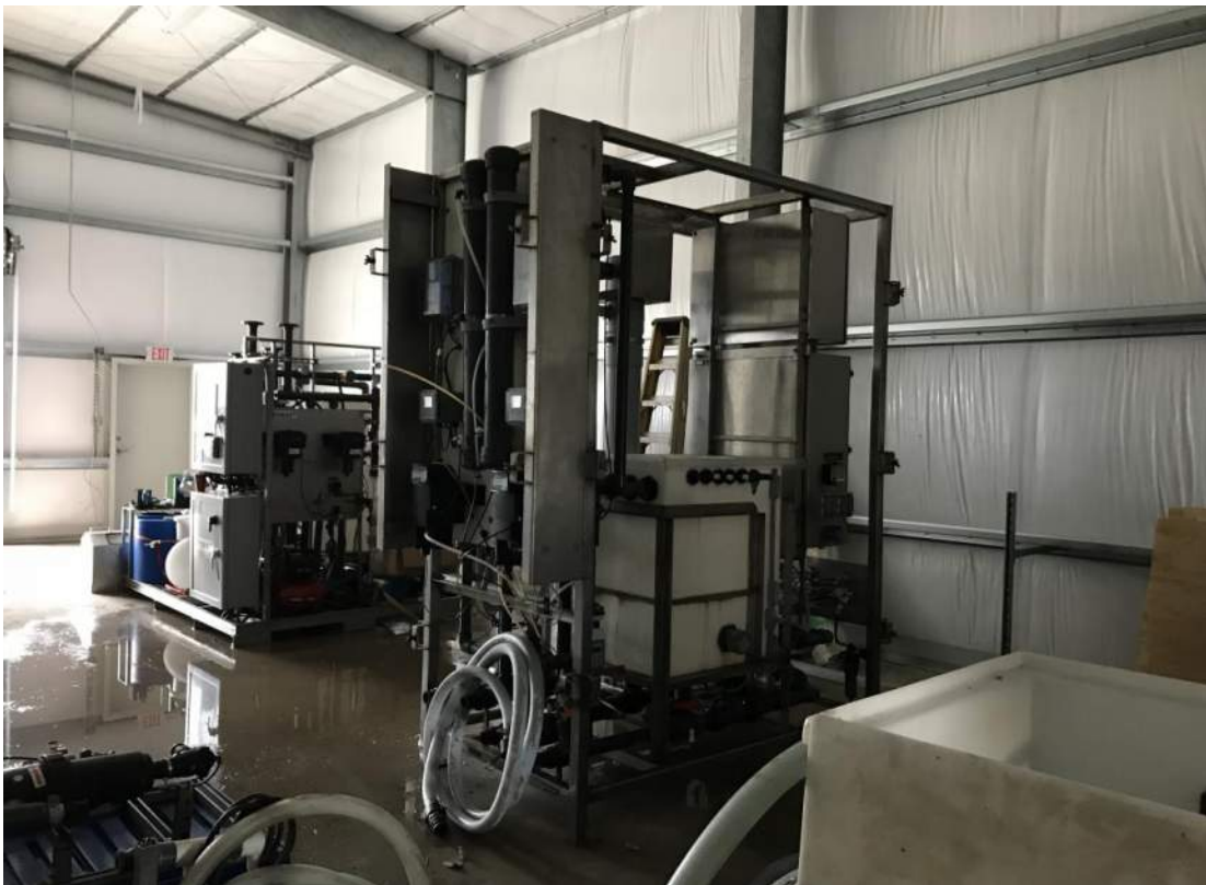
Membrane Filter Units - Toray, Evoqua, and Pall
