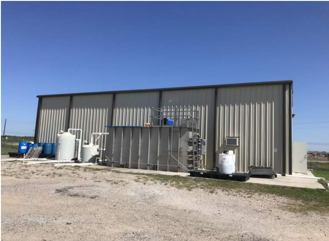
Raw Water Flocculation and Plate Settlers
