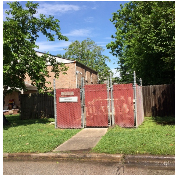
Orange-Mykawa Lift Station
