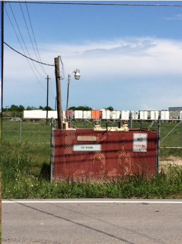
Shank Lift Station
