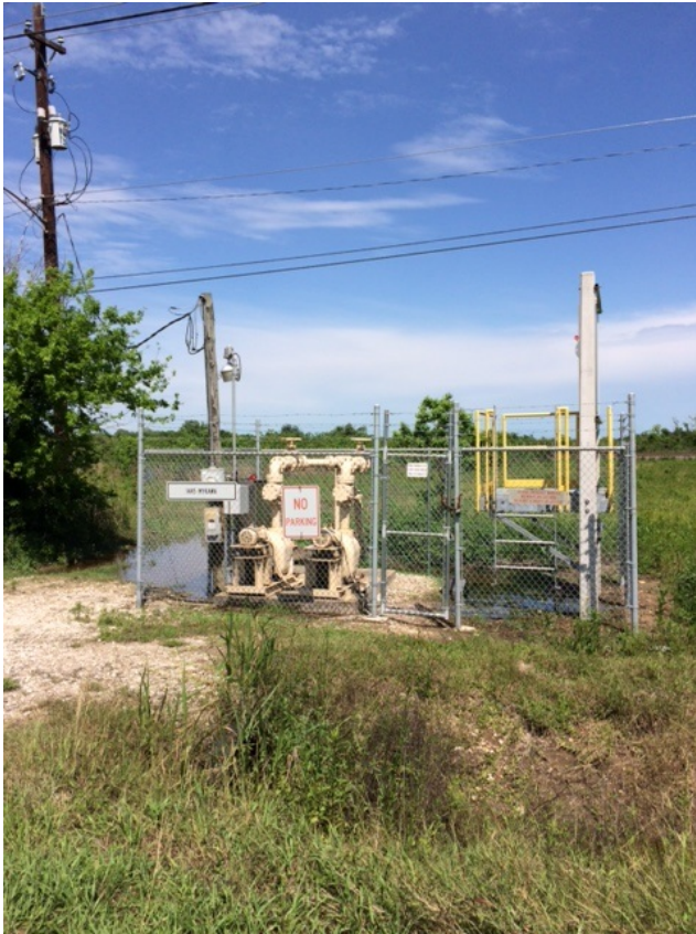
Mykawa-Scott Lift Station
