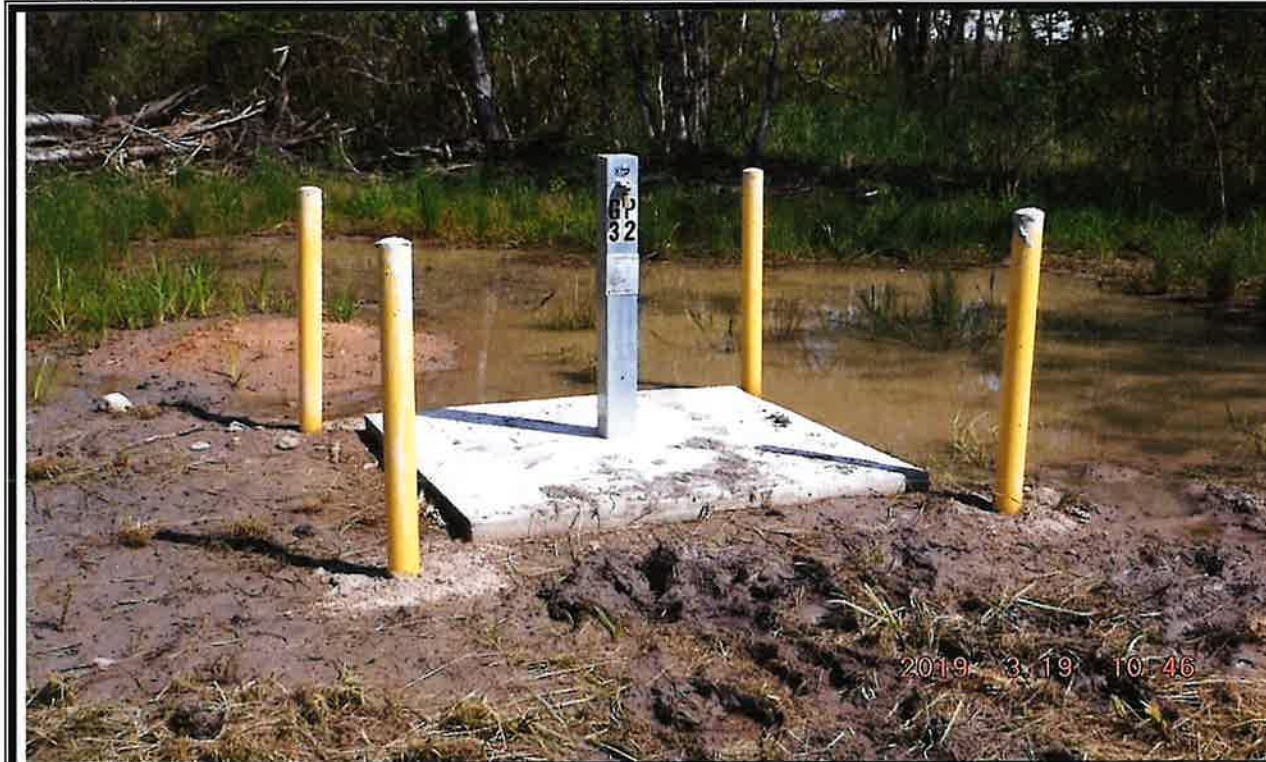
Photo No. 1 Gas Monitoring Probe GP-32. Permanent probe was locked, well supported, protected and maintained.
