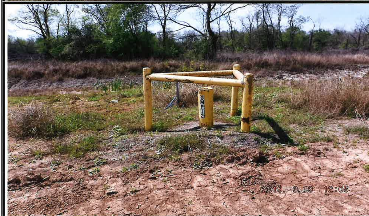
Photo No. 2 Gas Monitoring Probe GMP-12. Permanent probe was locked, well supported, protected and maintained.
