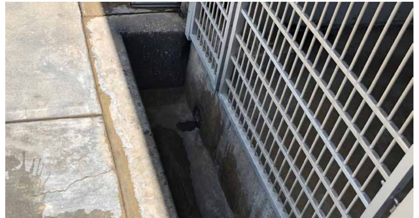
Exterior - Outdoor Runs - Open Trench Drain
