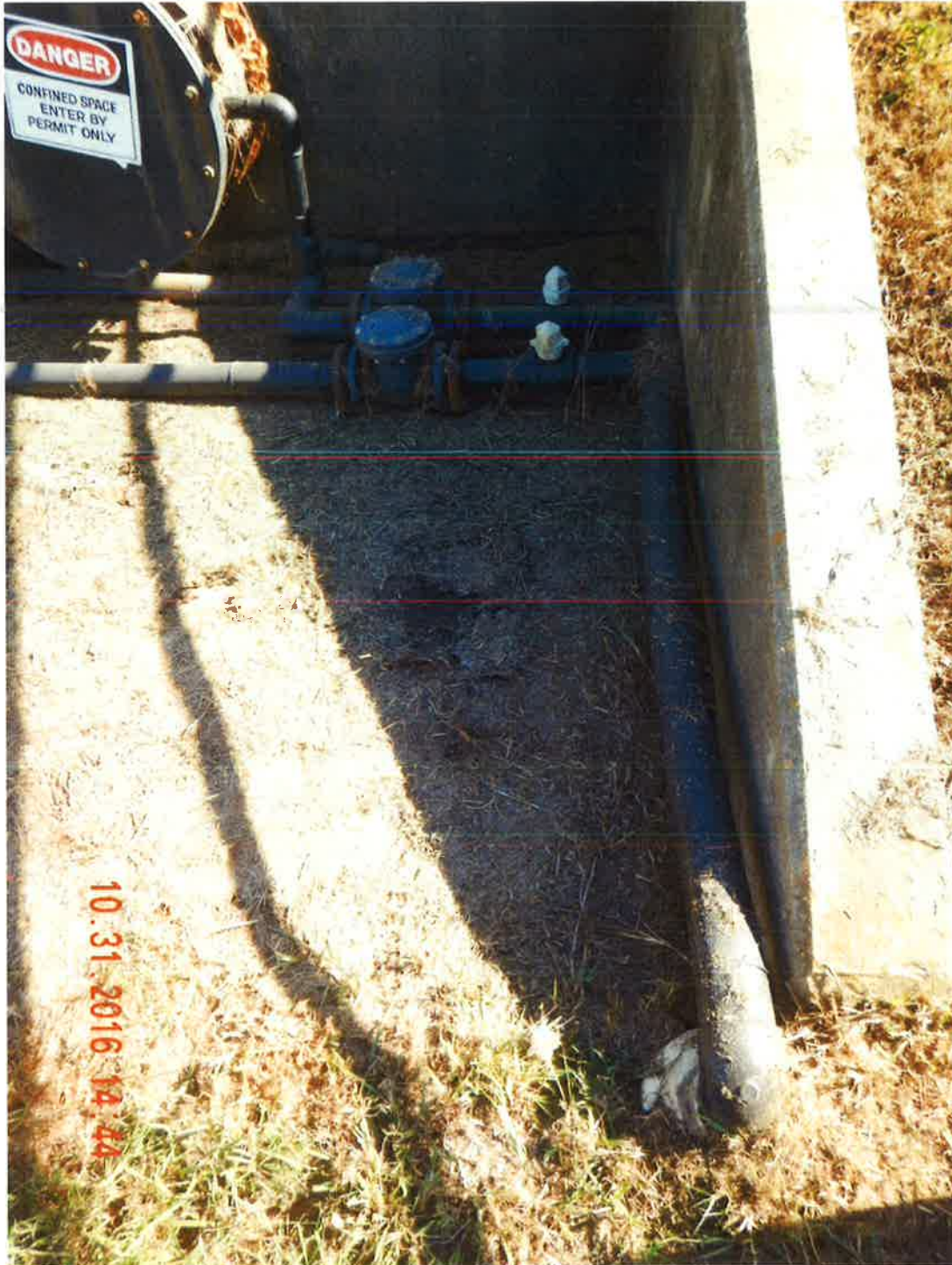
Photograph 2 of 2: Once the 2" pipe is outside of the 18" pipe headwall containment, it runs underground to reach the two leachate tanks.
