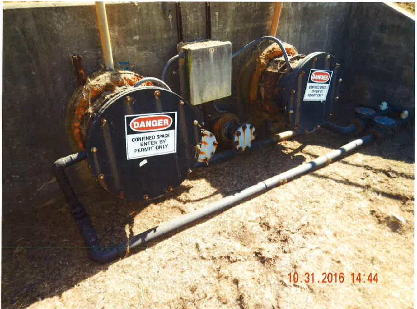
Photograph 1 of 2: Two 18" riser pipe ends visible at the sideslope of the landfill. Between them, two 6" cleanout riser pipe ends are visible. 2" pipes emerge from the 18" pipe headwall containment and run along the ground.
