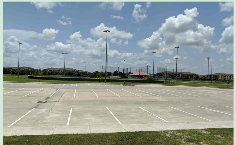
Current condition of Parking at The Sports Complex at Shadow Creek Ranch.
