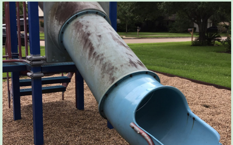
Current condition of Play Equipment at Corrigan Park.
